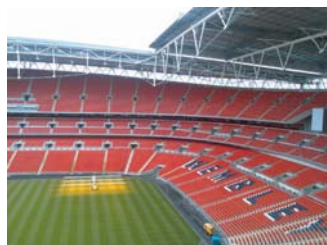
Fig. 2.3.11.A Artificial lighting rig in operation at Wembley stadium
