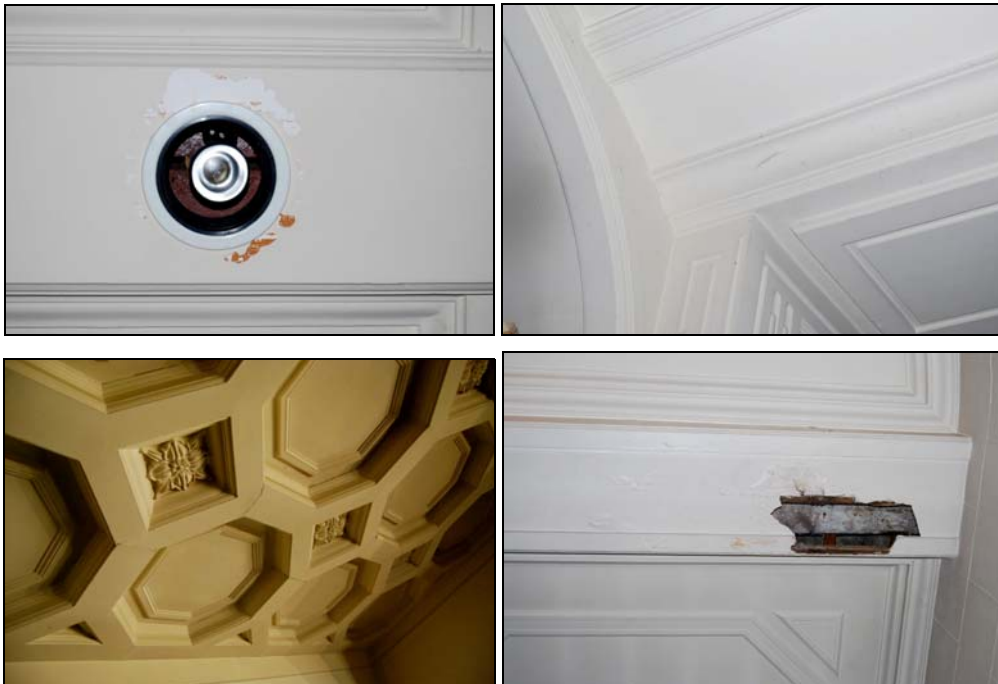
Typical plasterwork details showing (clockwise from top left): Insertion of modern light fitting, with peeling paint revealing original terracotta paint beneath; hairline cracking and crazing; cracks along joins in heavier moulded pieces, missing section of plasterwork surrounded by damp staining.
