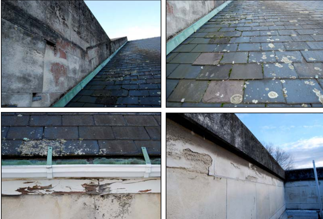
Roofing details showing (clockwise from top left): Delaminated stone and damp staining to north parapet; Lichen growth to slate surfaces; Damage to timber fascia; Delamination and salt growth to south parapet
