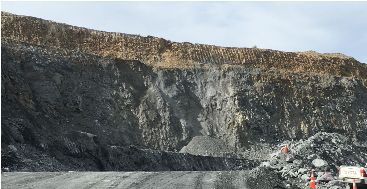
Photo 5: Coronation Pit Stage 2 – eastern wall of the ‘southern limb’. The 22.5 m high batters have not performed well in this rock mass.
