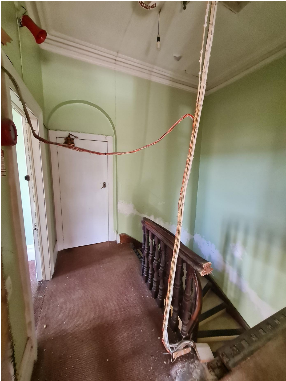
Photo 3 - Exposed electrical wiring, upper level
