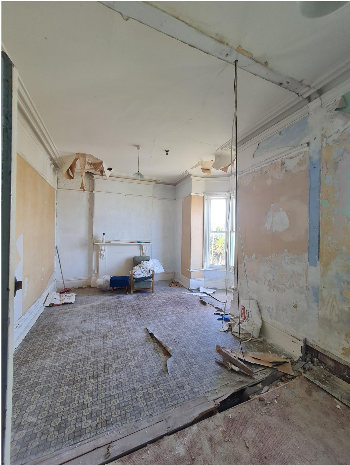
Photo 4 - Removed wall with no additional bracing or support & exposed electrical wiring, upper level
