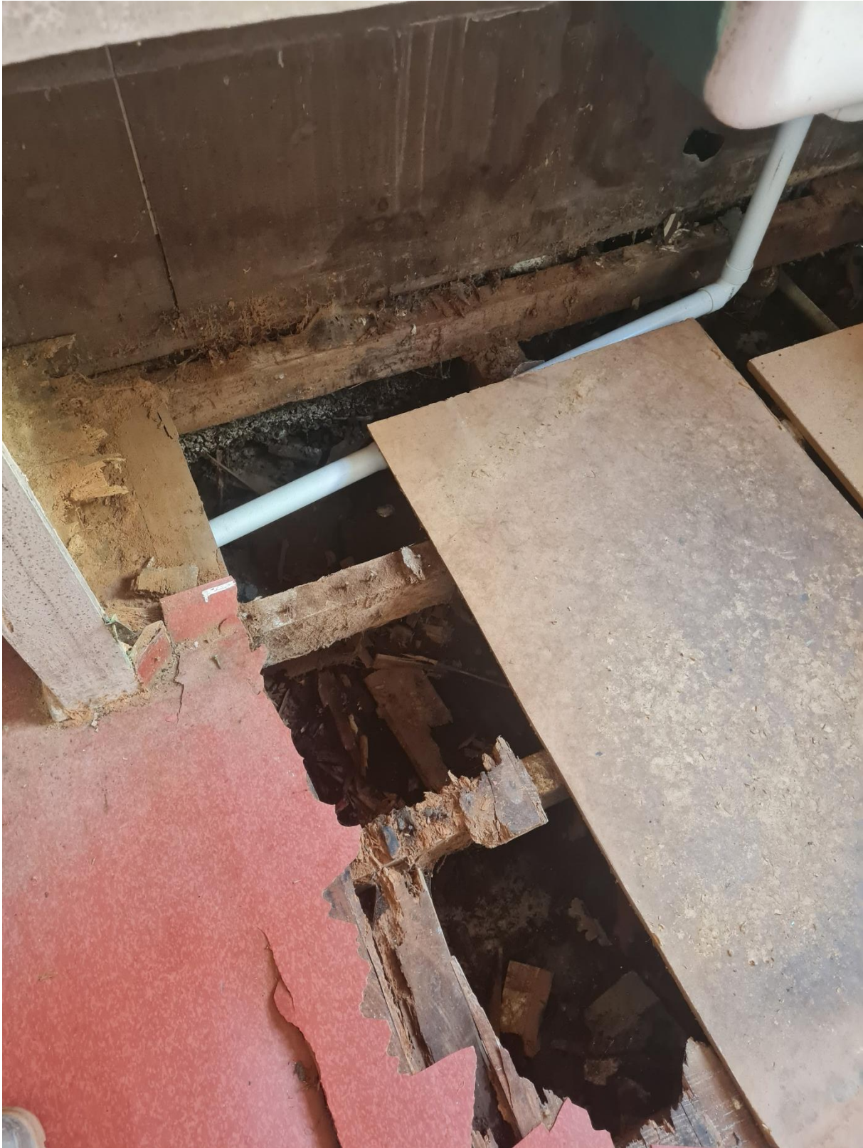
Photo 6 - Rotted floor framing, ground floor
