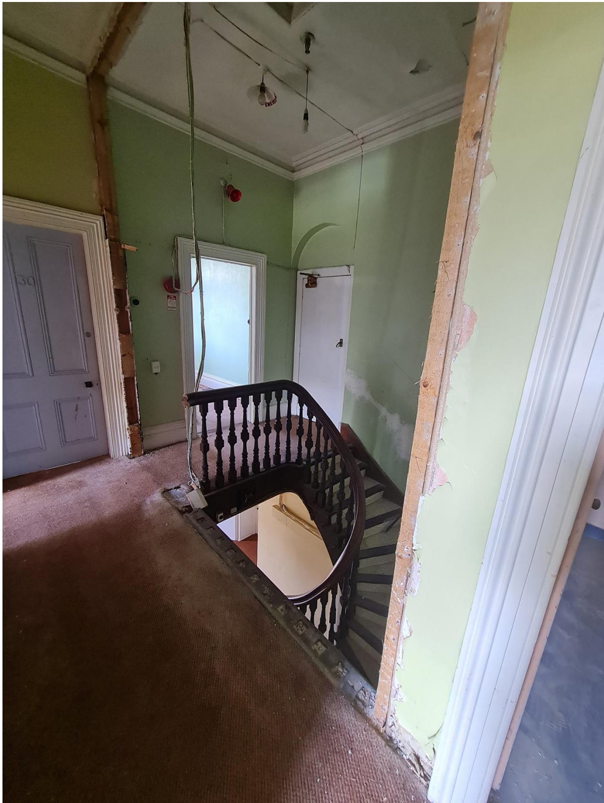
Photo 2 - Removed wall / fall hazard at stair shaft
