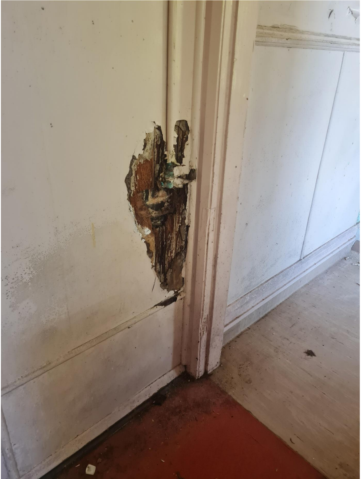
Photo 5 - Water damage, ground floor wall
