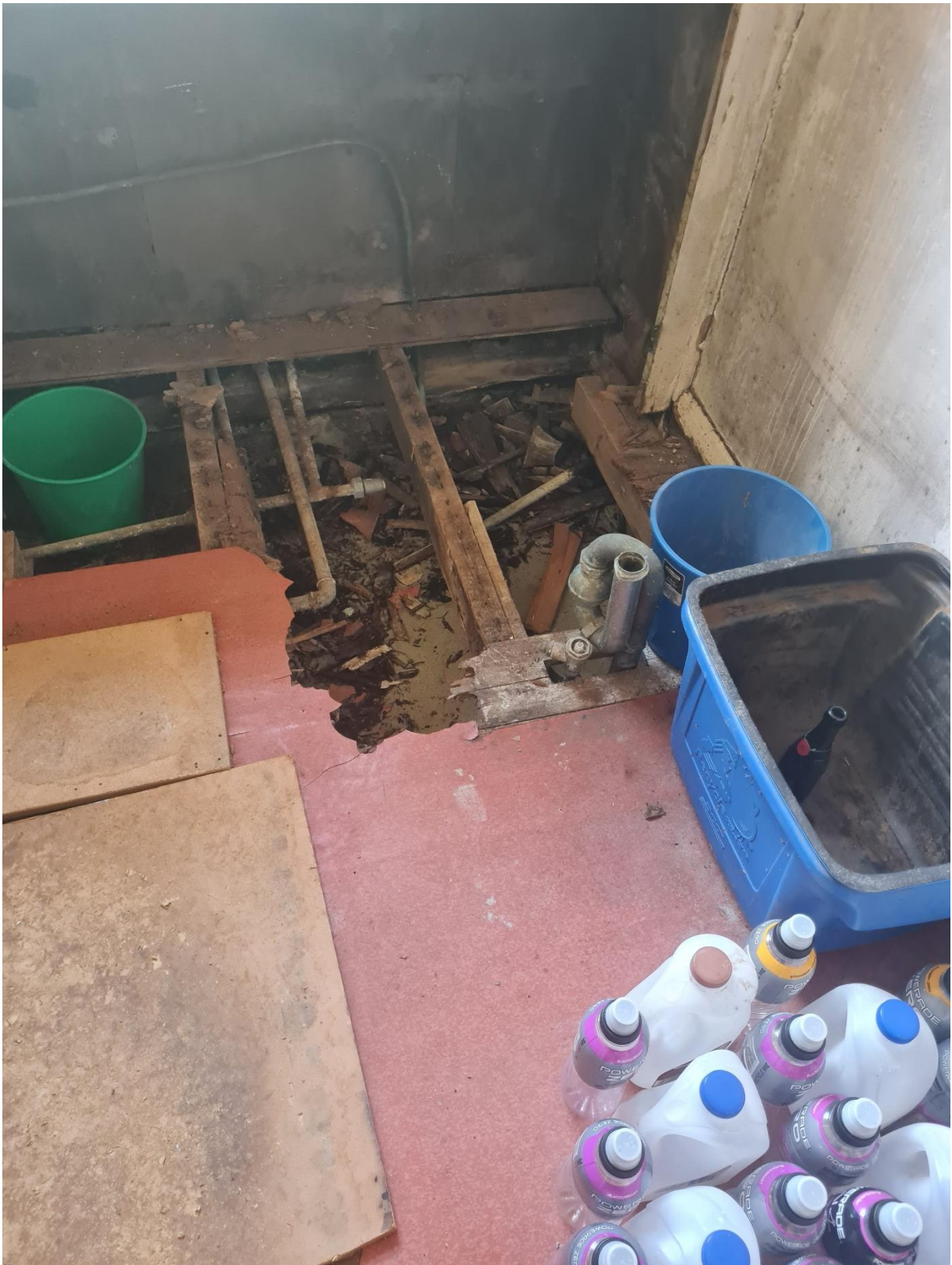
Photo 1 - Rotted floor framing bearing directly on soil
