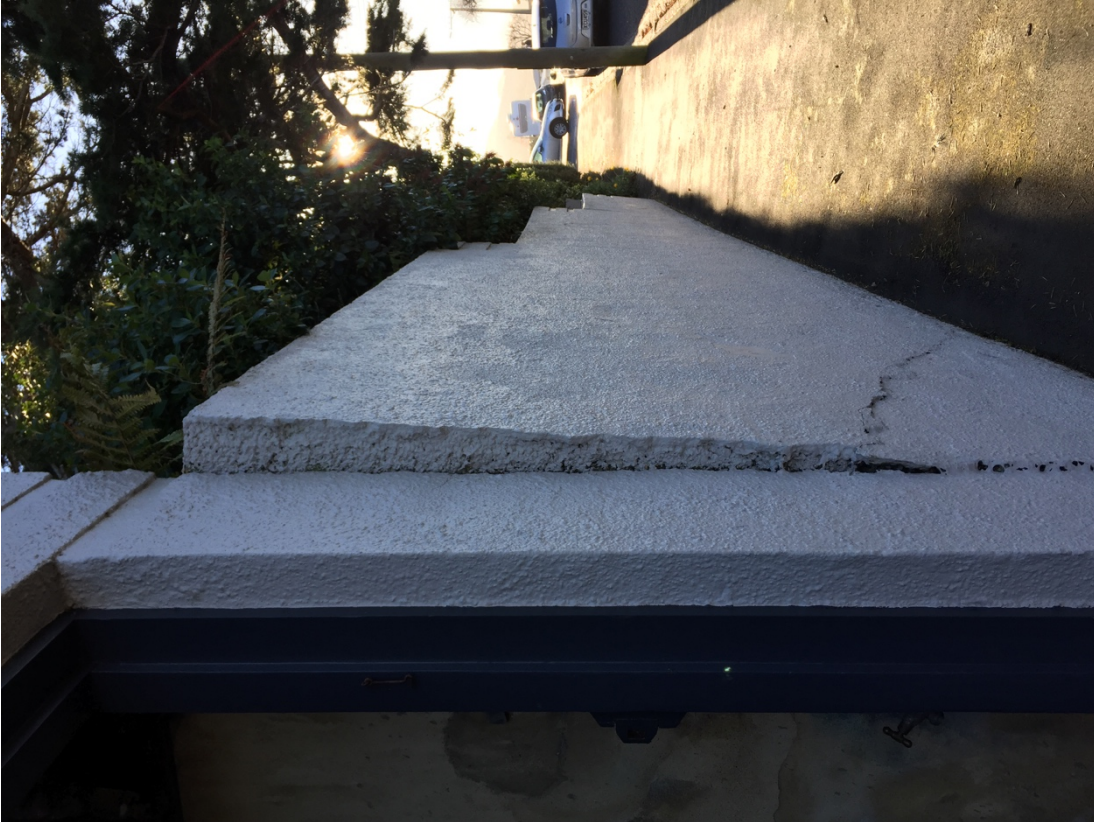
Image three: Image showing the front boundary fence / retaining wall at number 27 Falkland Street leaning out towards the footpath
