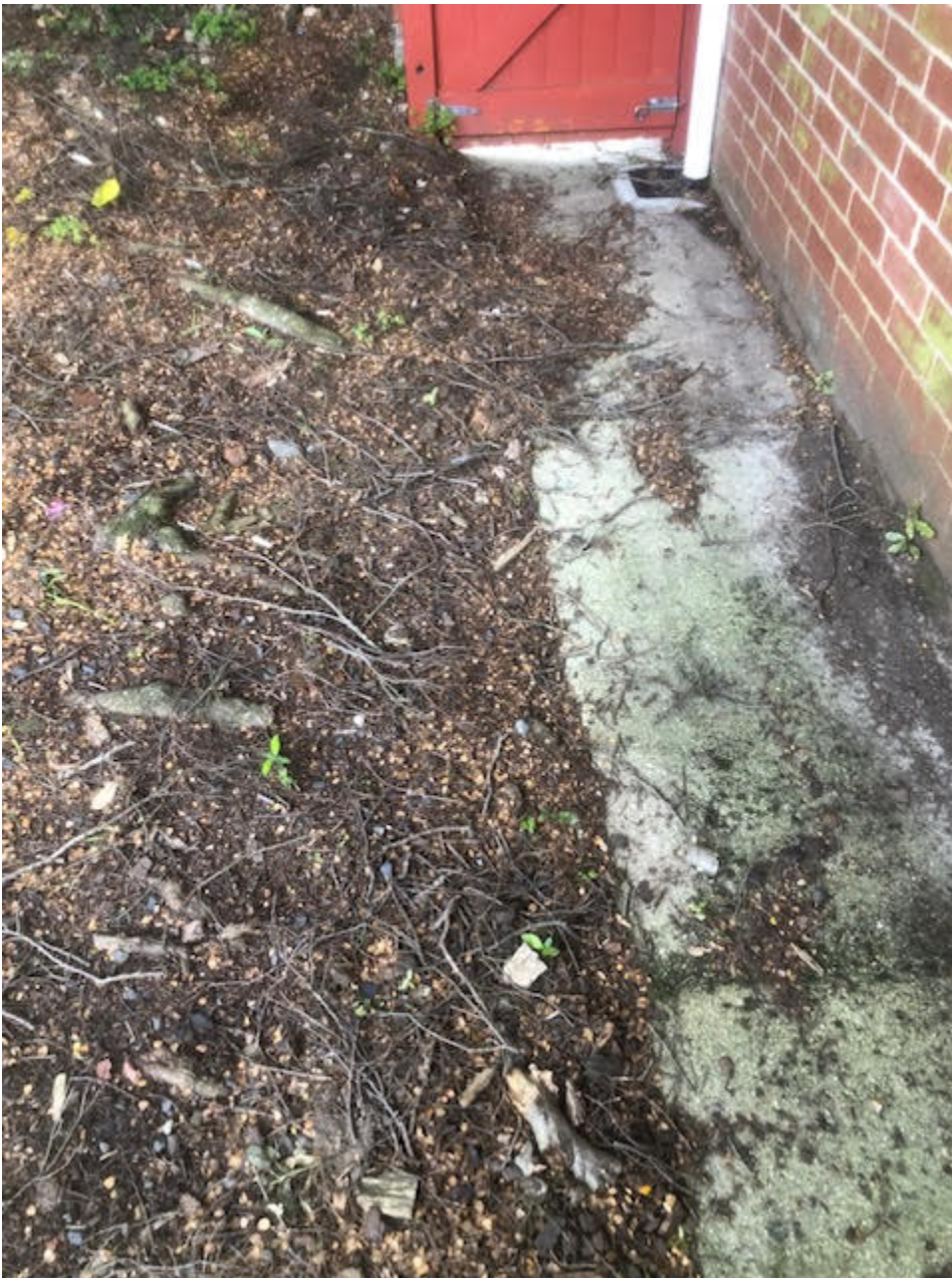
Figure 3 showing exposed roots
