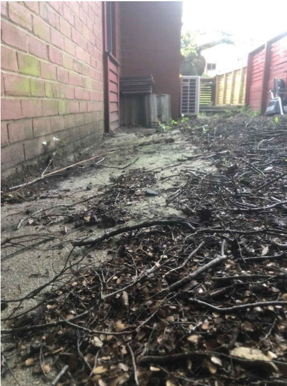
Figure 4 showing the uneven footpath next to the house where there are roots present
