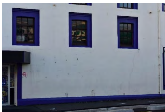
Figure 17: External view of the façade wall to Block 1 showing plaster cracks and damp at pavement level.
