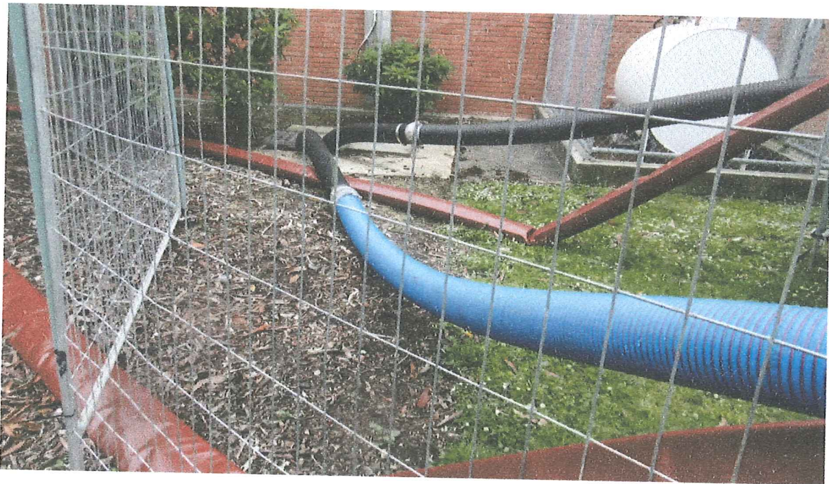
January 2021 Auxiliary Pumps Required at Portobello Road Pump Station, also in moderate rainfall (Issues not fixed ?)
