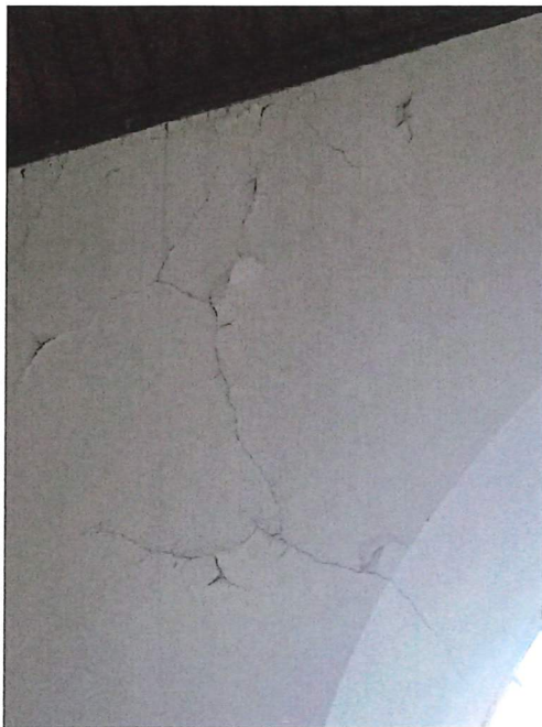
Internal: Water Egress Damage & Toxic Mould.
