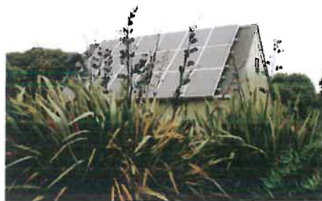
Figure 23 Roof-mounted PV array
