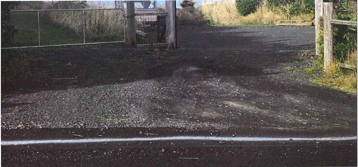
View of access formation. Note signs of edge break and gravel migration.
