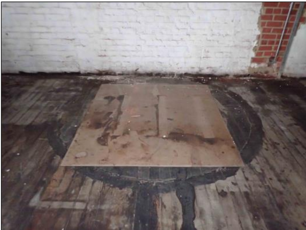
Figure 7-27 Photograph looking north at circular floor stain and covered floor in former kiln building.
