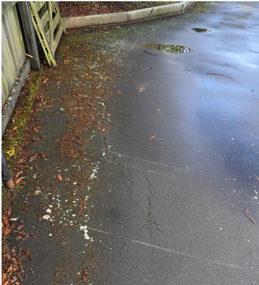
Figure 8: Existing cracks and undulation in driveway 27a Riccarton Road East next to TX002.
