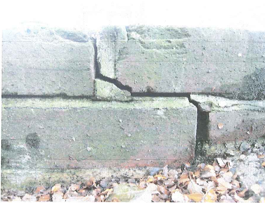
Photo 2. Crack at 1 in photo 1. Also evident is the 20mm elevation of the concrete slab to the right, which now impedes drainage from the drive.
