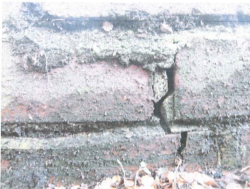
Photo 3. Crack at location 2 in photo 1.
