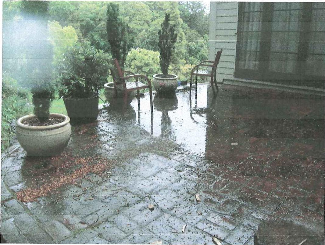
Photo 8. Ponding of water on patio, caused in part by elevation of left side of patio by tree roots.
