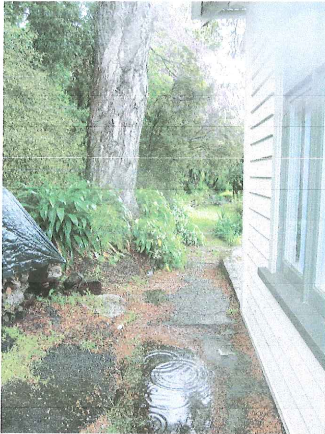
Photo 7. Ponding of water draining from drive, impeded by elevation of concrete slab beneath the tree.
