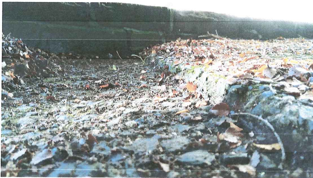
Photo 6A & B. Ponding of drainage from drive caused by 20mm elevation of concrete slab at bottom of picture (6B).
