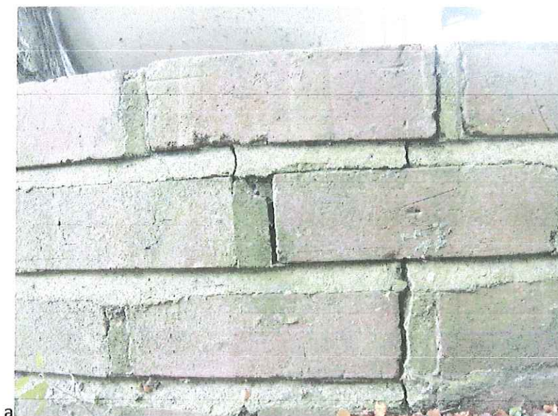
Photo 4. Crack at location 3 in photo 1.
