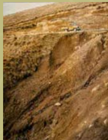
LARGE SLIP, 1980 FLOODS
