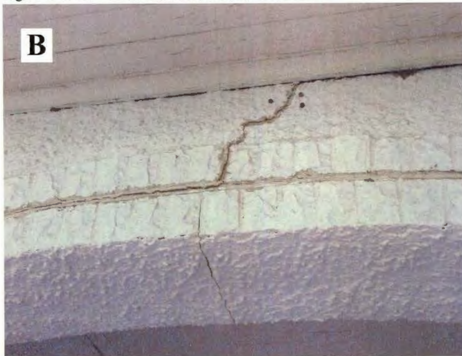
Figure 5. Crack in arch above front door, location B
