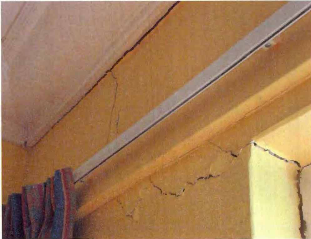
Figure 10. Internal cracking near ranch-slider door (corresponding to external location E)
