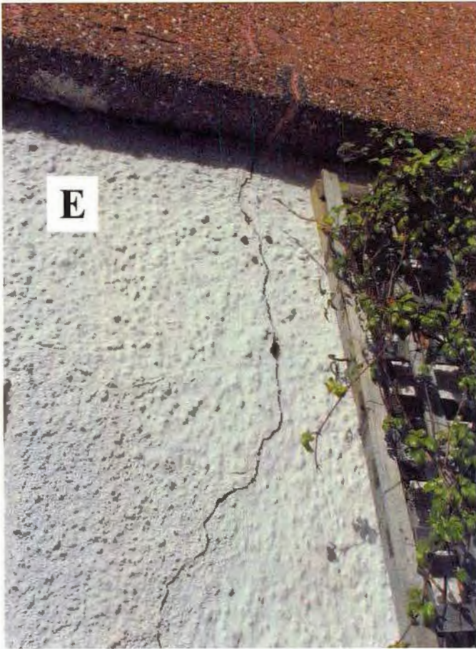
Figure 9. Crack next to ranch-slider at location E
