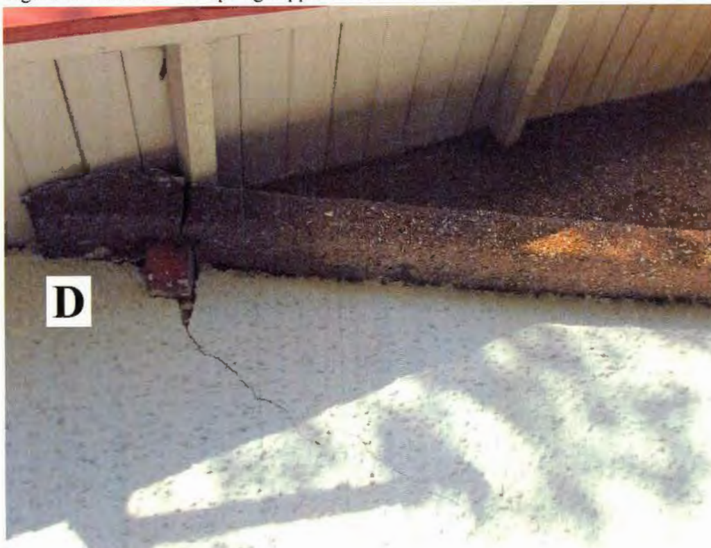
Figure 8. Crack and collapsing support at location D corner
