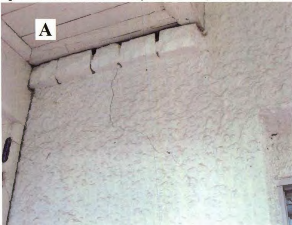
Figure 4. Crack in wall at the corner of porch, location A (north west corner)
