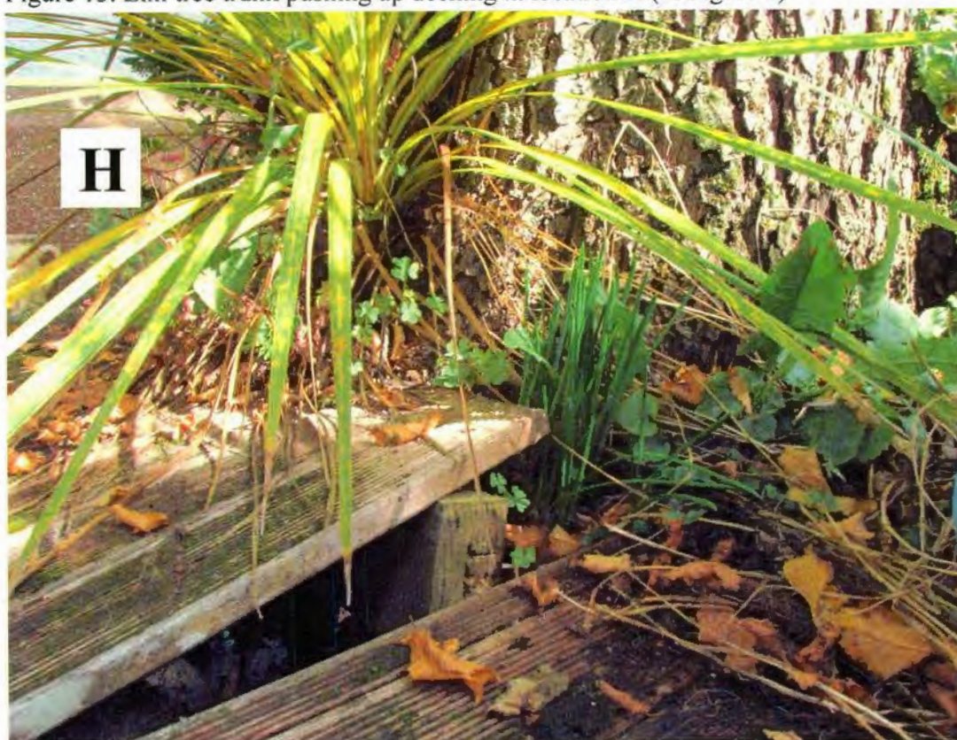
Figure 13. Elm tree trunk pushing up decking at location H (in Figure 7)
