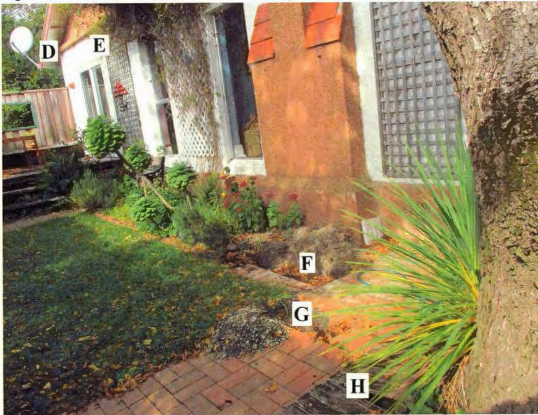
Figure 7. Location of cracks – north side of house
