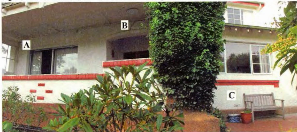
Figure 3. Location of cracks – front of house facing Grater Street
