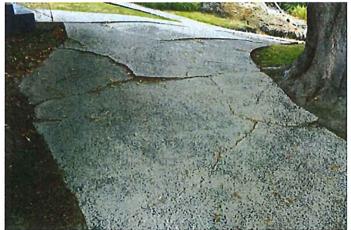
Broken concrete on driveway and car park area.
