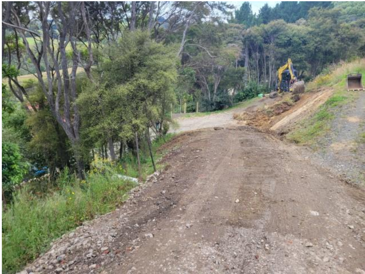
Photograph 3: Landslide debris and some fill removed from outside road shoulder, with minimal (recent) fill remaining to be removed
