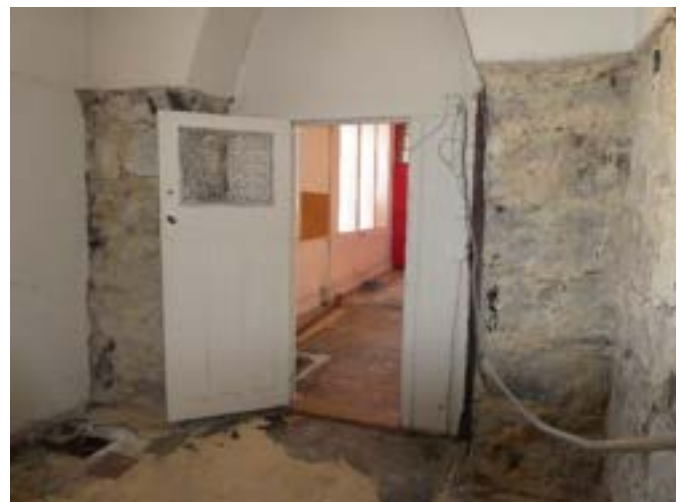
Photograph 153 - Showing the plaster removed from the basement administration office.
