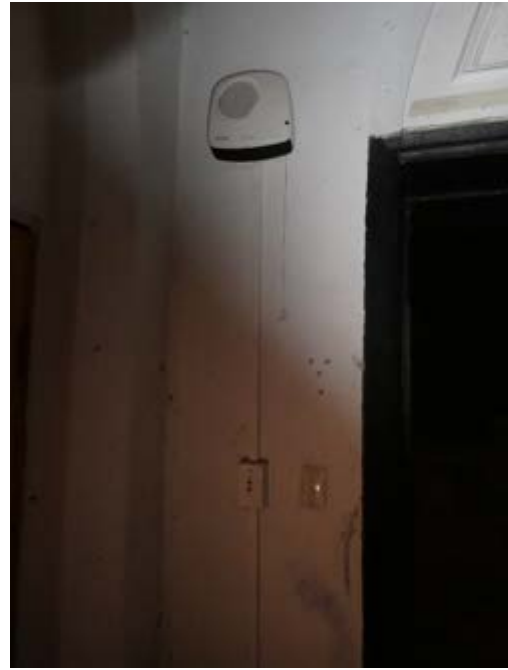
Photograph 260 – Showing the electric fan heaters adjacent to the main theatre entrances.
