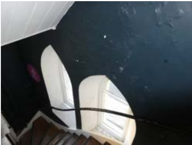
Photograph 154 - Showing the defective plasterwork above the timber lancet windows to the south eastern stair.
