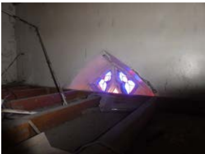
Photograph 67 - Showing the ceiling joists and the hidden top to the leaded lancet window within the roof space above the kitchen / bar.
