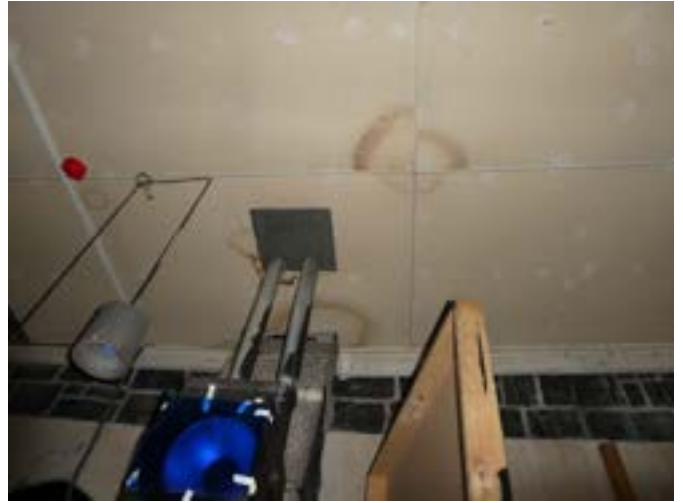
Photograph 125 – Showing the moisture stained ceilings to the now enclosed south western area adjacent to the main stage..
