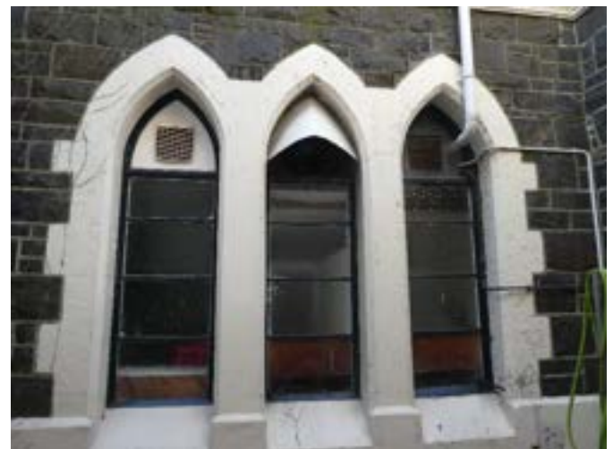
Photograph 51 – Showing the steel framed windows on the western elevation. Noting inappropriate positioning of services.
