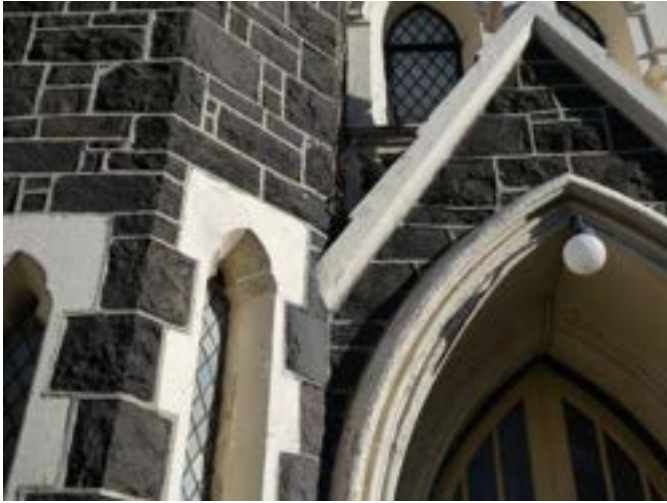
Photograph 31 – Showing the vegetation growth above the northern entrance.
