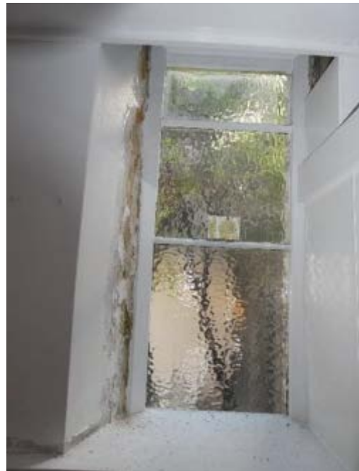
Photograph 185 – Showing the defective paint and plaster to the window in the south western toilets.
