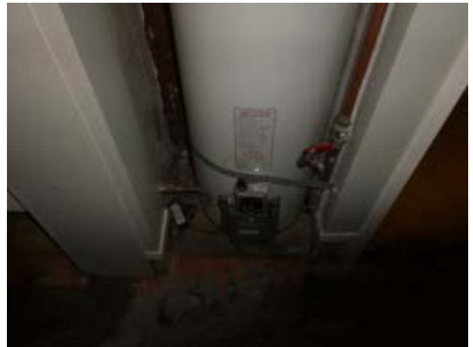
Photograph 251 – Showing the mains pressure gas hot water cylinder housed within the basement toilets.
