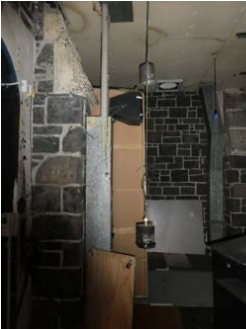
Photograph 88 - Showing the exterior walls to the now enclosed area to the south western corner. Noting moisture staining to the ceiling linings.
