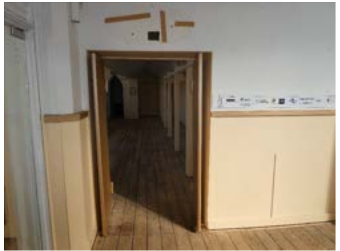
Photograph 76 – Showing the double doors leading from the entrance foyer to the bar.
