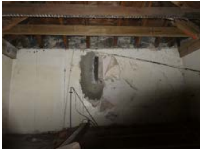
Photograph 66 – Showing the paint failure to the hidden walls within the roof space above the kitchen / bar.
