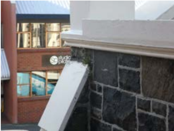
Photograph 37 - Showing the vegetation growth to the north western buttress.
