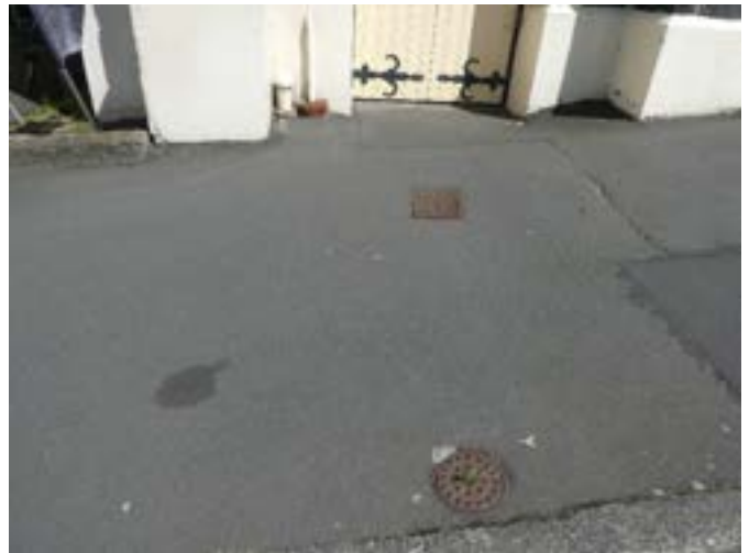
Photograph 248 – Showing the water shut off point to the south east.
