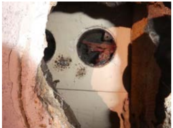
Photograph 247 – Showing old redundant VIR cables within the internal walls.
