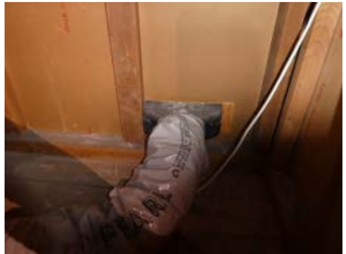
Photograph 258 – Showing the insulated warm air ducting below the seating with outlet to the bar area.
