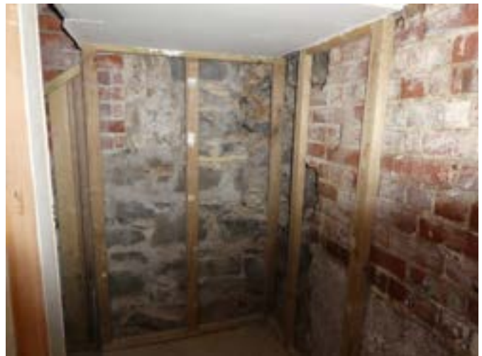
Photograph 200 – Showing the linings removed from the basement floor to the former project managers office at the north western stairwell.
