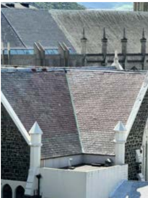
Photograph 13 – Showing the south western roofs and flat roof area above the extension.
