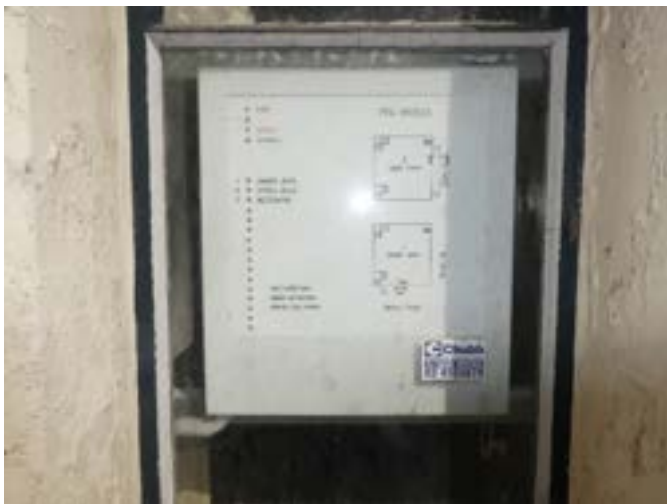
Photograph 240 – Showing the fire alarm panel on the eastern elevation.
