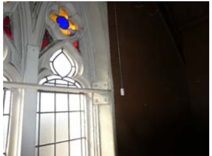
Photograph 167 – Showing the horizontal steel reinforcing / strengthening bar to the inside of the mullioned window. Noting cracking to the stone surround.
