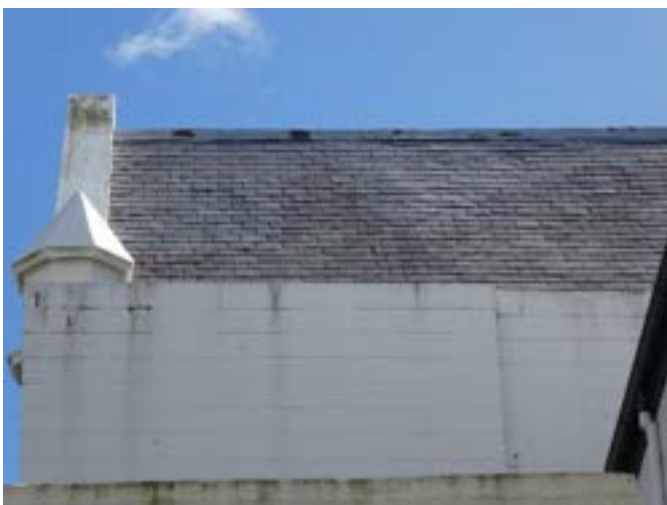
Photograph 3 – Showing the south western roofs and flat roof area above the extension.
