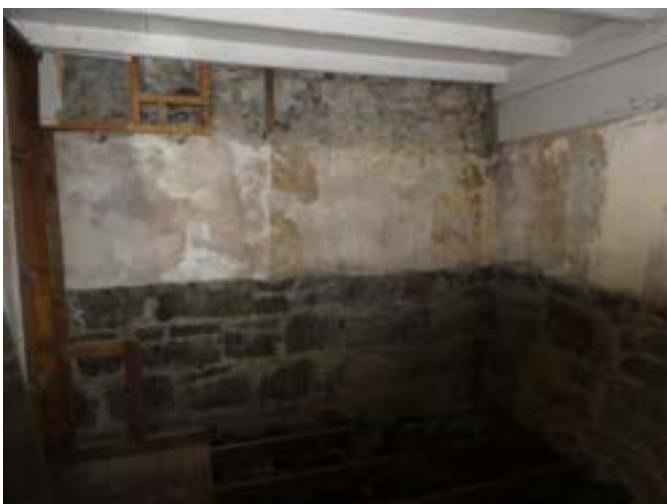
Photograph 108 - Showing the unlined / plastered walls to Dressing Room 2 accessed off the Green Room.
