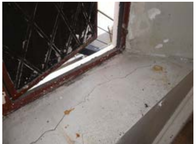
Photograph 179 – Showing the defective cracked plasterwork to the steel leaded lancet windows at the stair landing on the western elevation.
