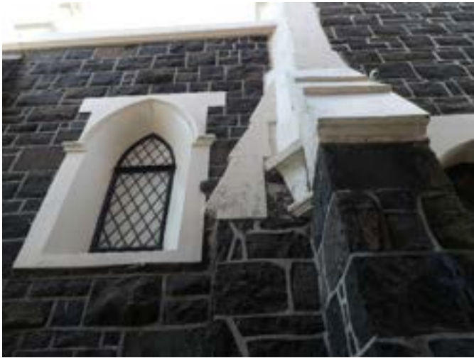
Photograph 60 - Showing the leadlight lancet window and buttress to the north eastern elevation.
