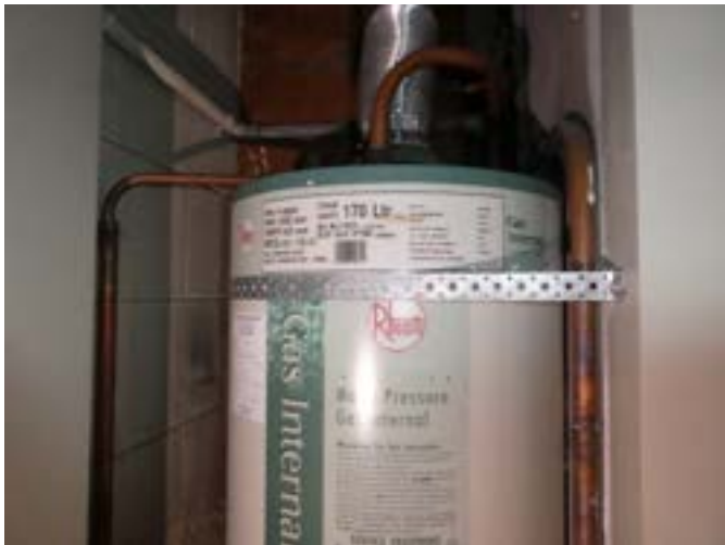
Photograph 250 – Showing the mains pressure gas hot water cylinder housed within the basement toilets.
