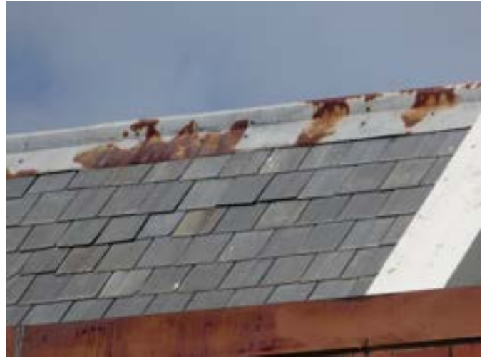
Photograph 6 – Showing the corroded ridge flashings to the north.
