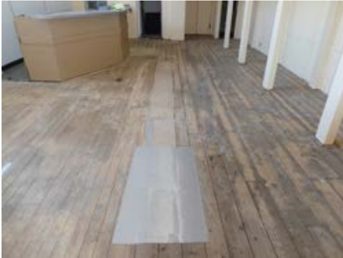
Photograph 133 - Showing the timber floor boards and target repairs within the bar area.
