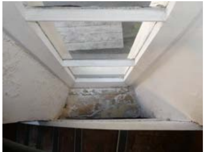
Photograph 155 – Showing the defective plasterwork to the sill of the timber lancet windows to the south eastern stair.
