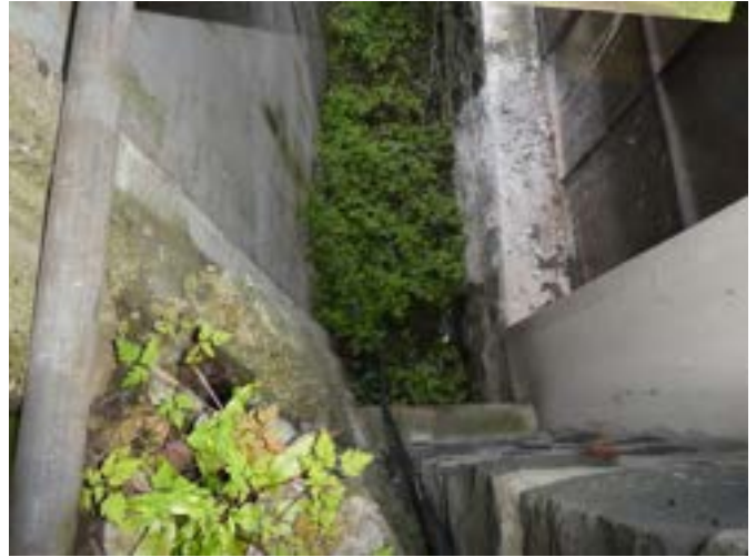
Photograph 234 – Showing the concrete retaining wall to the south western elevation.
