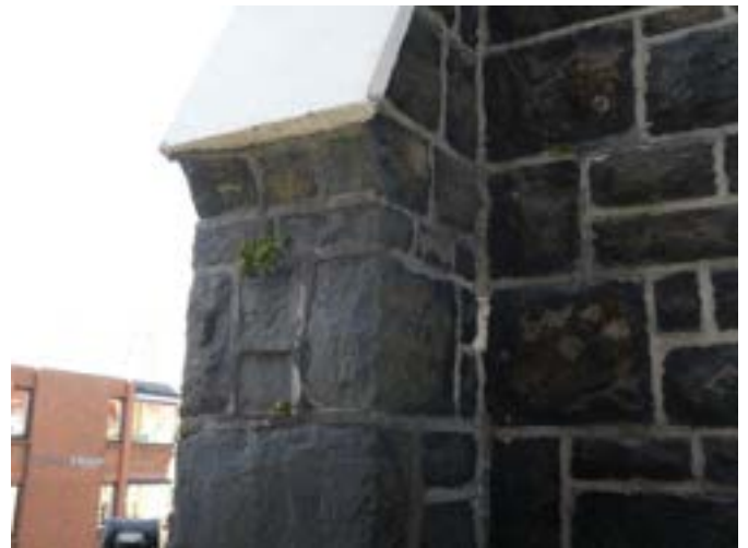
Photograph 36 – Showing the vegetation growth to the north western buttress.
