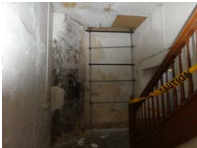
Photograph 202 – Showing the temporary propping within the north western stairwell. Noting unidentified blackspot mould to the plaster walls
