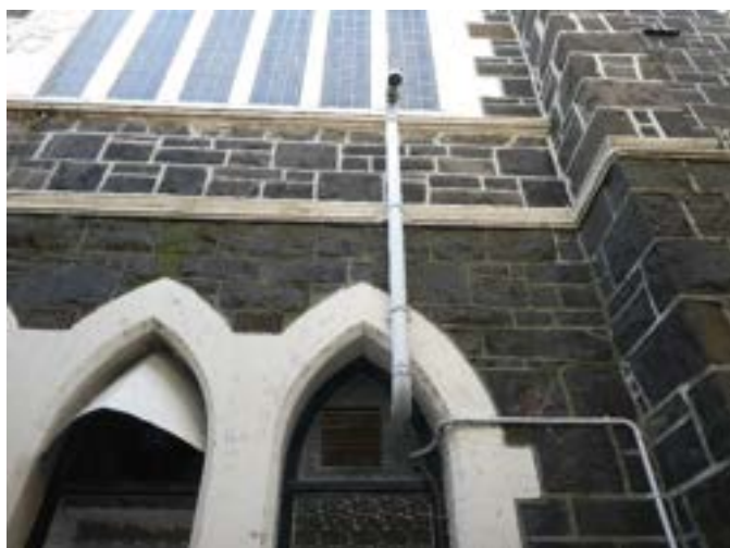
Photograph 54 - Showing the steel framed windows on the western elevation. Noting inappropriate positioning of services.
