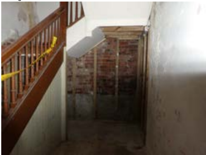
Photograph 199 - Showing the linings removed from the basement floor to the former project managers office at the north western stairwell.
