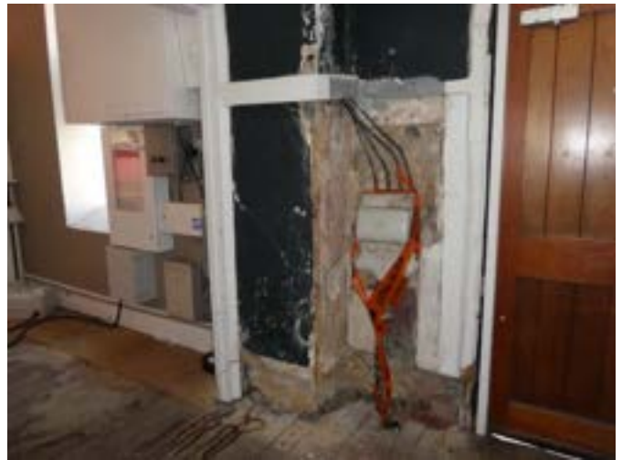
Photograph 244 – Showing the old electric meter.
