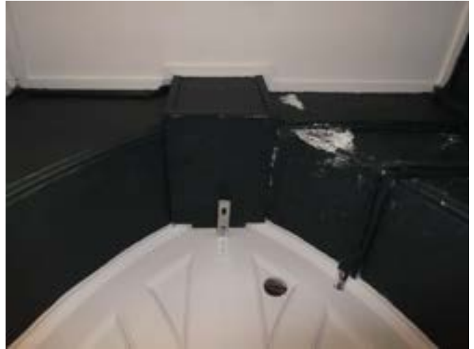
Photograph 193 – Showing the condition of the timber infill panel above the internal doorway to the basement foyer. Noting efflorescence to the solid walls
