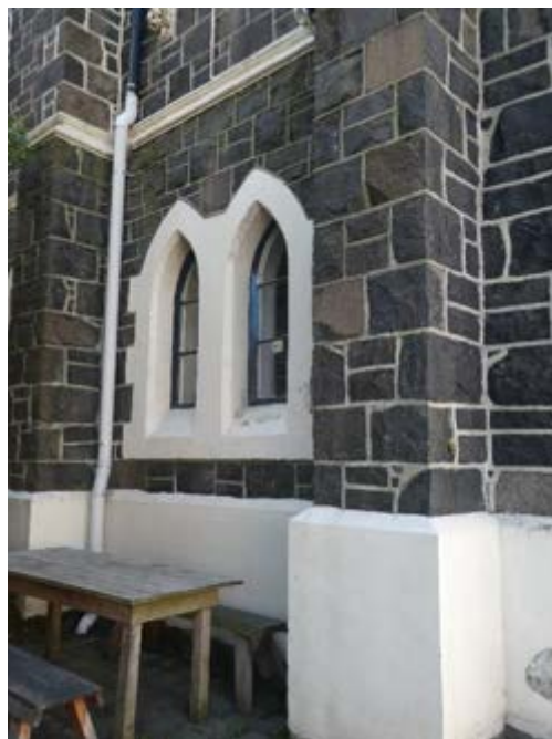
Photograph 53 – Showing the steel framed windows to the south western courtyard area. Noting paint failure, and replacement putty.
