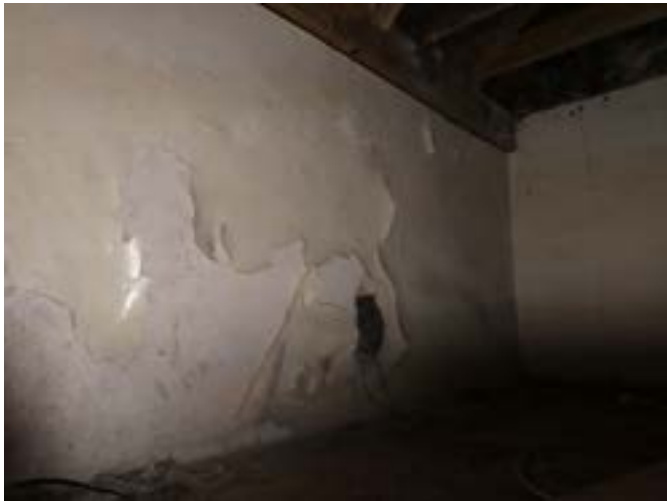
Photograph 65 - Showing the paint failure to the hidden walls within the roof space above the kitchen / bar.
