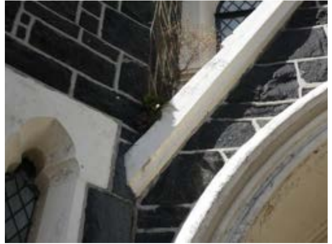
Photograph 32 – Showing the vegetation growth above the northern entrance
