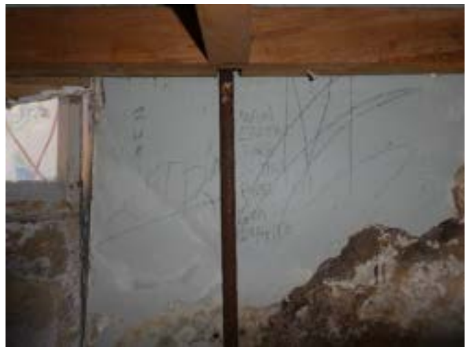
Photograph 165 – Showing the typical condition of the basement walls below the south eastern stairs.
