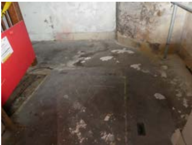
Photograph 197 - Showing the basement floor to the former project managers office / stairs at the north western stairwell.
