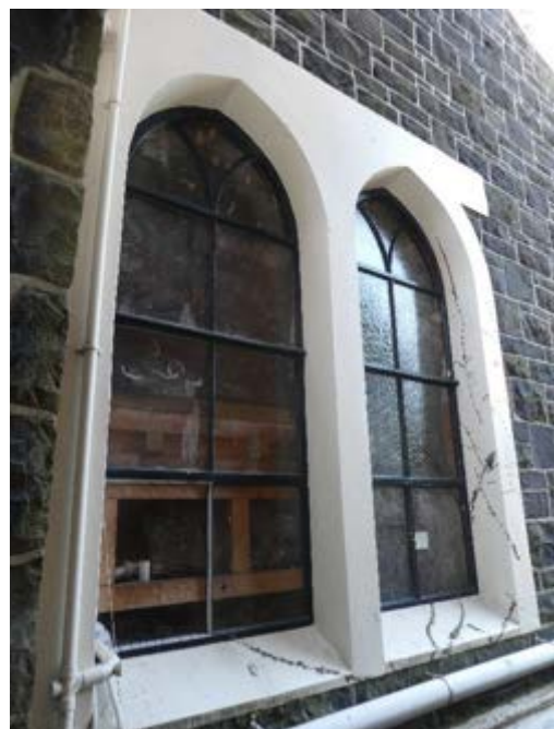
Photograph 63 – Showing the western elevation. Noting corrosion to the steel window frame
