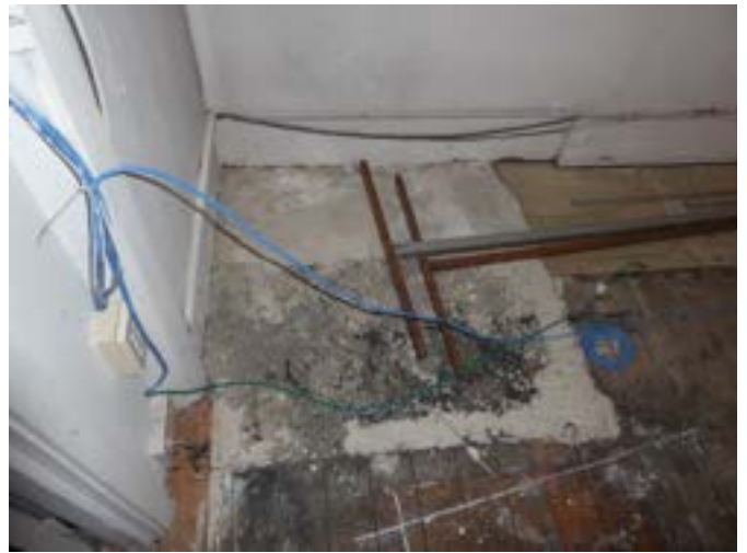
Photograph 142 – Showing the piecemeal repairs to the basement office floor noting concrete, timber and custom wood.
