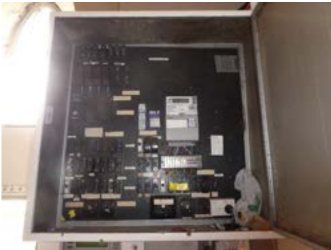
Photograph 243 – Showing the main switchboard to the south eastern basement foyer.
