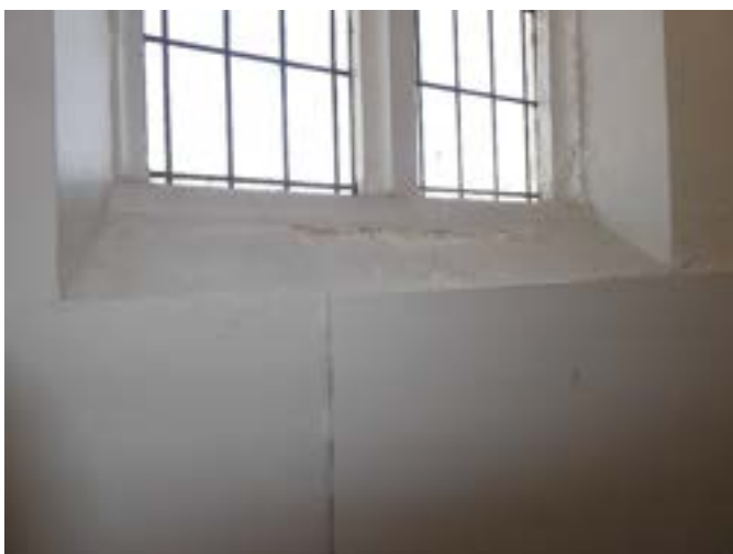
Photograph 180 – Showing the defective paint and plaster to the window sill on the southern wall.
