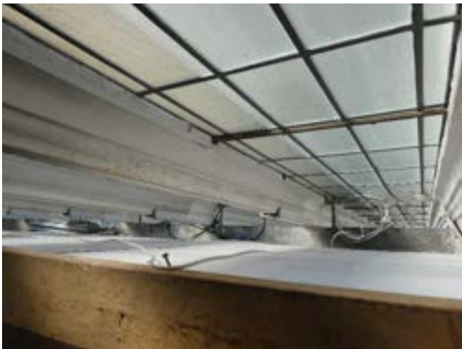
Photograph 168 - Showing the corroded horizontal steel reinforcing and strengthening bars to the inside of the mullioned window.
