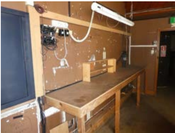
Photograph 145 - Showing the damaged fibrous plaster wall and benching to the meeting / theatre technical room.
