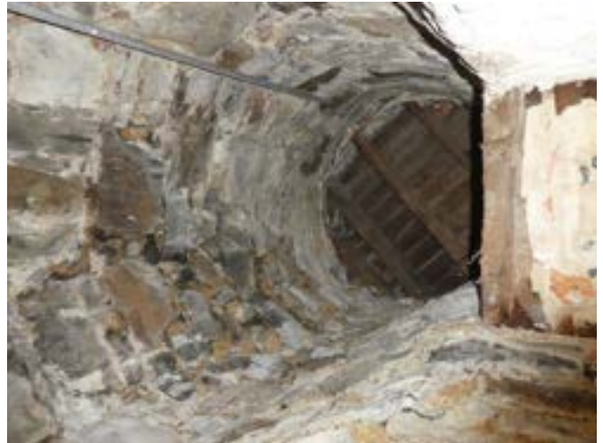
Photograph 161 – Showing the ceiling / timber floor installed within the bell tower looking up from the basement area.
