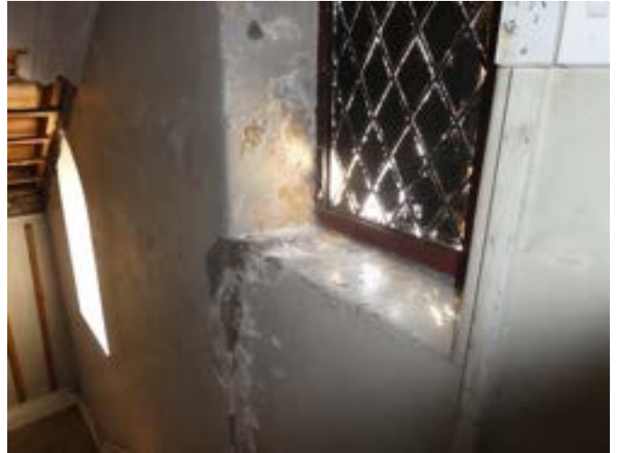
Photograph 177 – Showing the defective plaster and efflorescence to the jamb and sill of the steel leaded lancet windows at the stair landing on the eastern elevation.
