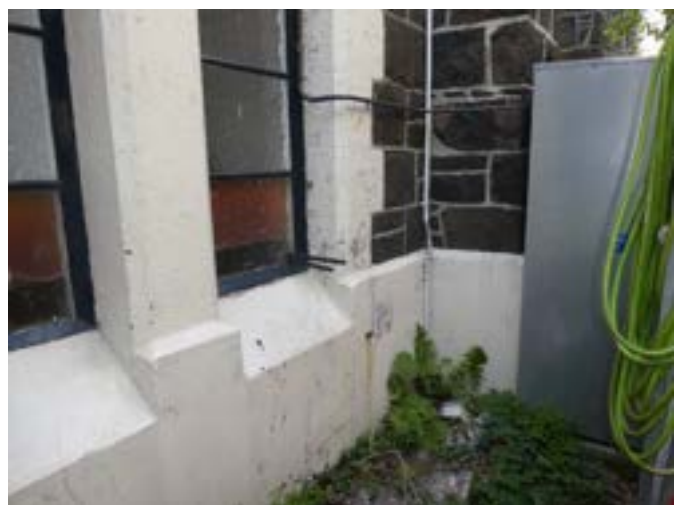
Photograph 239 – Showing the vegetation growth to the southern courtyard area.
