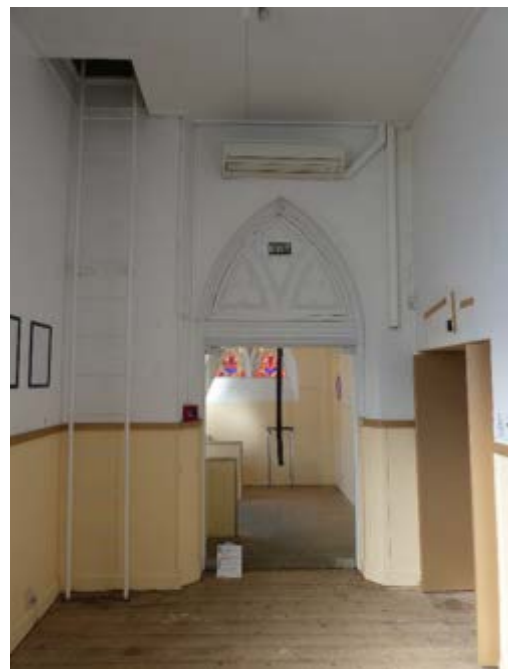
Photograph 242 – Showing the vertical fire escape ladder from the meeting / theatre control room to the entrance foyer.
