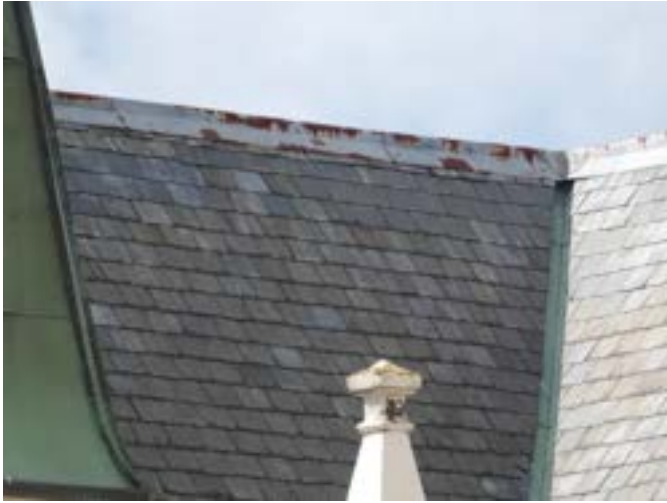
Photograph 5 – Showing the corroded ridge flashings to the north.
