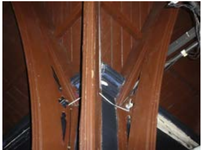
Photograph 196 – Showing the typical timber detailing at the base of the timber trusses at the columns within the main theatre.
