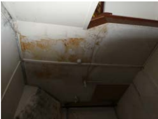
Photograph 203 - Showing the damage and staining to the ceiling linings within the north western stairwell.
