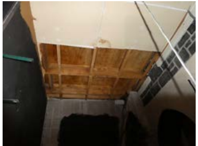
Photograph 64 – Showing the exposed and uninsulated flat roof to the south western extension.
