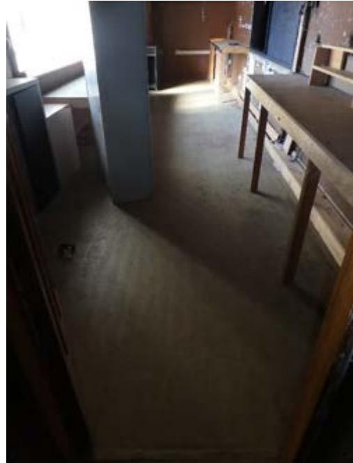
Photograph 130 – Showing the damaged vinyl flooring to the meeting / theatre technical room.
