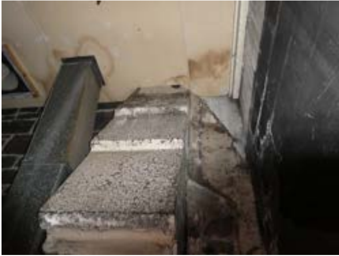
Photograph 124 - Showing the moisture stained ceilings to the now enclosed south western area adjacent to the main stage.
