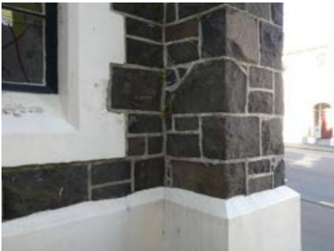
Photograph 35 – Showing the vegetation growth to the south eastern buttress.
