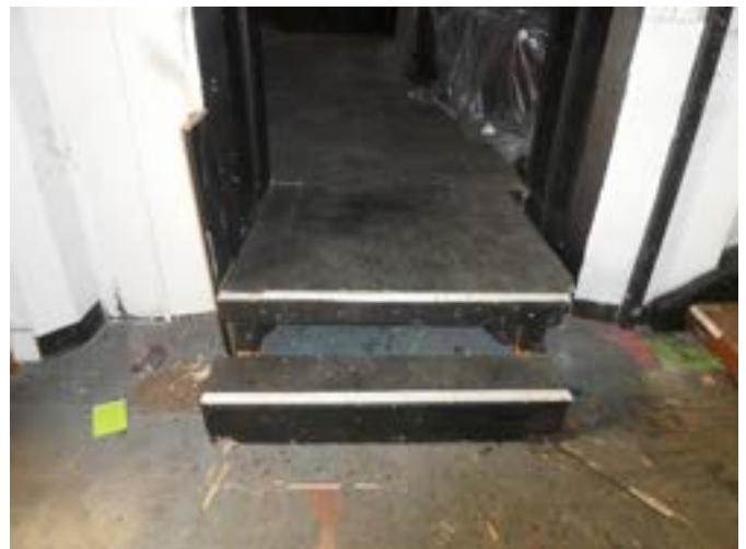
Photograph 191 – Showing the damaged steps leading to the main stage from stage left.
