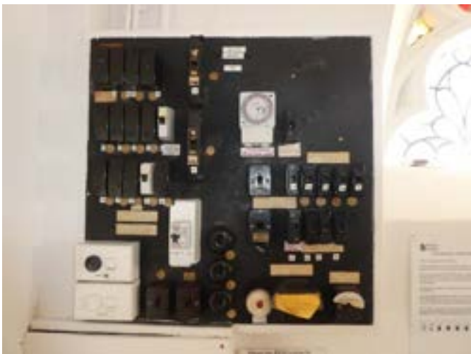
Photograph 246 – Showing the sub-distribution board to the bar / kitchen.
