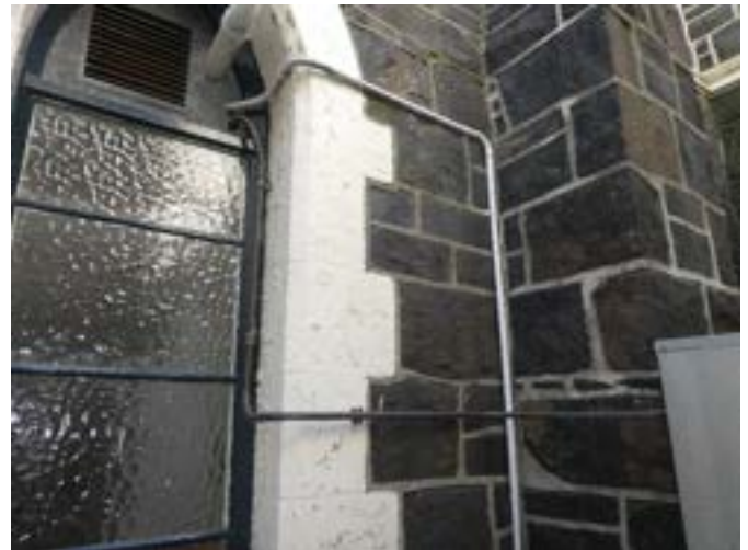
Photograph 262 – Showing the gas pipe penetration through the window.
