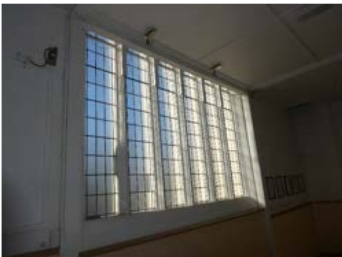
Photograph 170 - Showing the leaded windows and stone mullions at the base of the stained glass window to the east within the entrance foyer.
