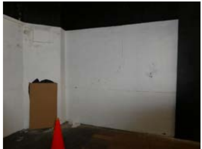
Photograph 151 - Showing the poor condition to the walls and opening within the studio theatre.
