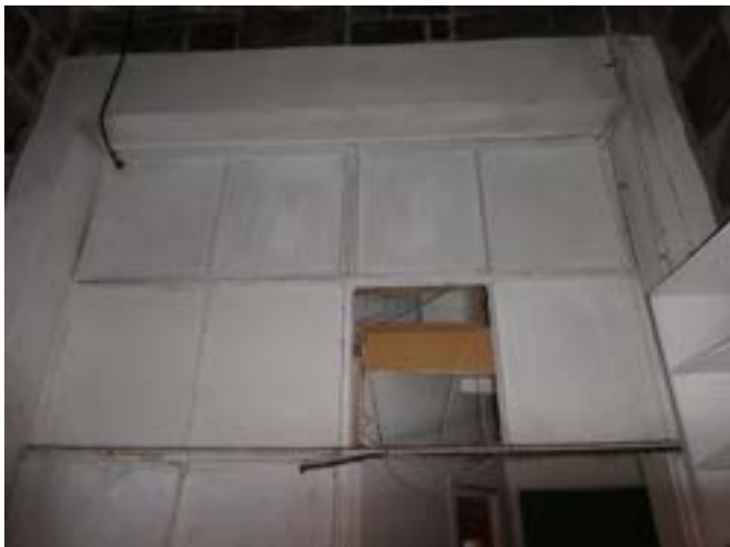
Photograph 186 - Showing the painted windows within the south western stairwell. Noting missing pane.
