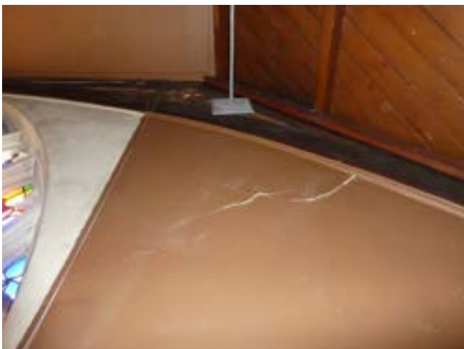
Photograph 147 - Showing typical hairline cracking to the plaster on the external walls.
