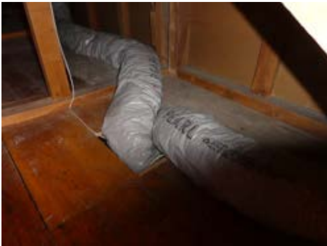
Photograph 257 – Showing the insulated warm air ducting below the seating in the main theatre.
