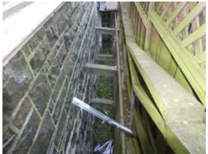
Photograph 236 – Showing the concrete braces buttressing the retaining wall to the western elevation.
