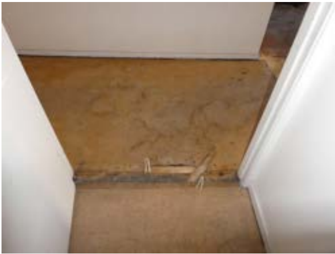
Photograph 141 - Showing the vinyl to the basement corridor and threshold to the male toilets.
