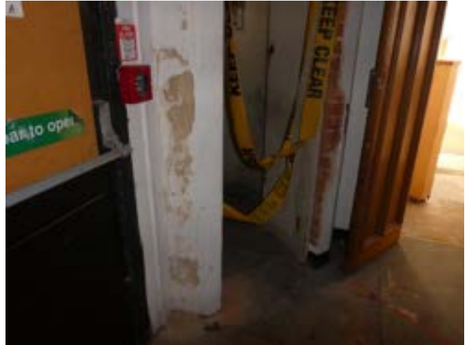
Photograph 159 – Showing the defective paint and plaster adjacent to the bell tower.
