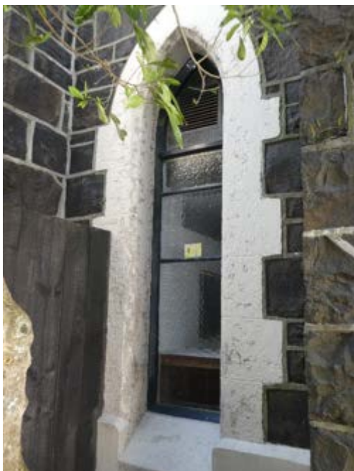
Photograph 52 - Showing the steel framed windows to the south western courtyard area. Noting paint failure and replacement putty.
