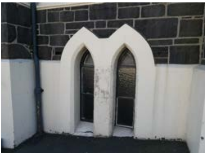
Photograph 56 - Showing the steel framed windows on the southern elevation. noting paint failure, cracking to the sill and unpainted replacement putty.
