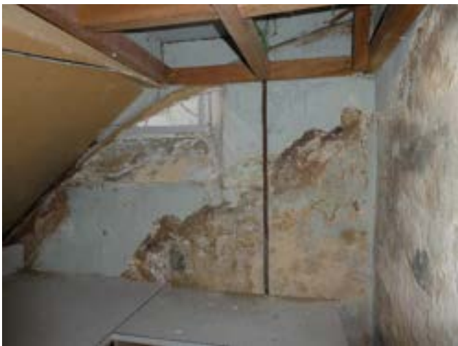
Photograph 164 - Showing the typical condition of the basement walls below the south eastern stairs.
