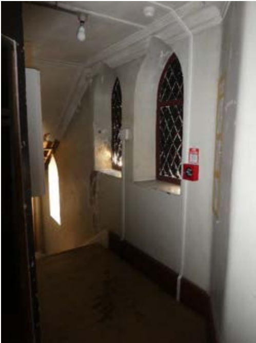
Photograph 176 - Showing the defective plasterwork to the steel leaded lancet windows at the stair landing on the eastern elevation.
