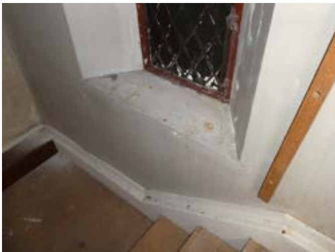
Photograph 178 - Showing the defective cracked plasterwork to the steel leaded lancet windows at the stair landing on the western elevation.
