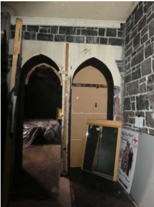
Photograph 90 - Showing the exterior walls to the now enclosed area to the south western corner. Noting the original steel sashes removed.
