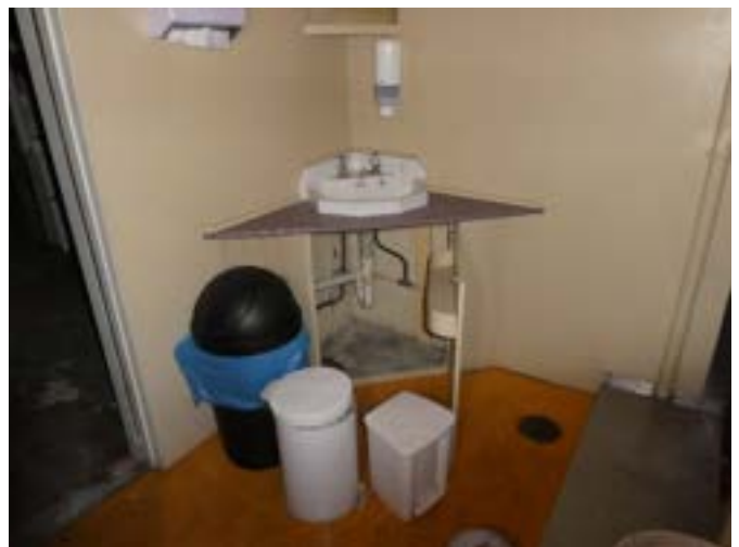
Photograph 219 – Showing the corner wash hand basin in the male toilet.
