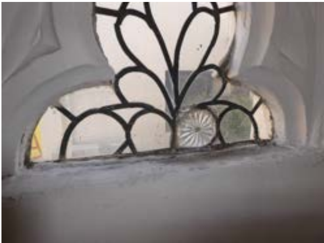
Photograph 174 - Showing inappropriate glazing repair and also noting cracking to glass panels.
