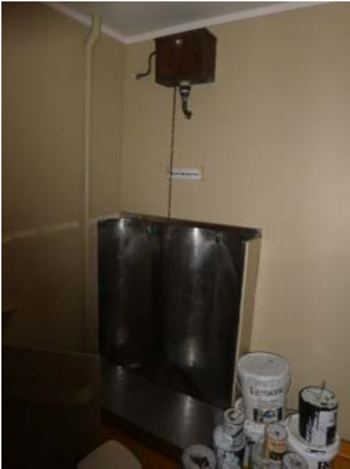
Photograph 220 – Showing the stainless steel urinal to the male toilet.
