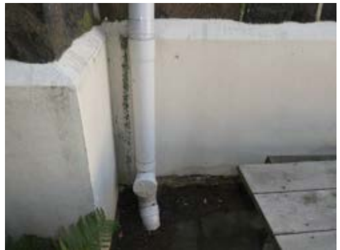
Photograph 19 – Showing the replacement uPVC rainwater downpipe and inspection point to the southern elevation.
