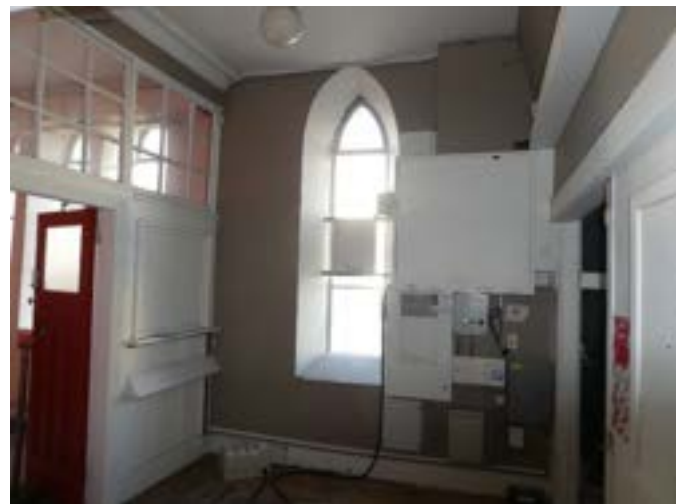
Photograph 241 – Showing the rear of the fire alarm panel within the basement.
