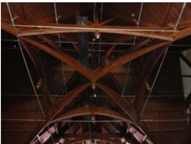
Photograph 122 - Showing the tie beams to the truss detail within the main theatre.
