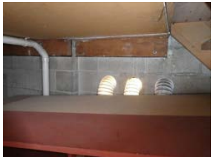
Photograph 252 – Showing the flexible ducting penetrations to the concrete masonry wall from the south western basement toilets.
