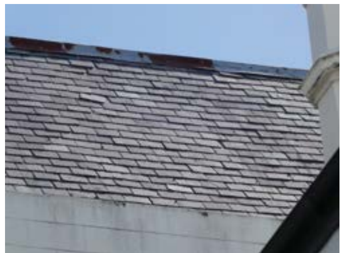
Photograph 4 – Showing the south western roof noting slipped slates and extensive rust to the ridge capping.
