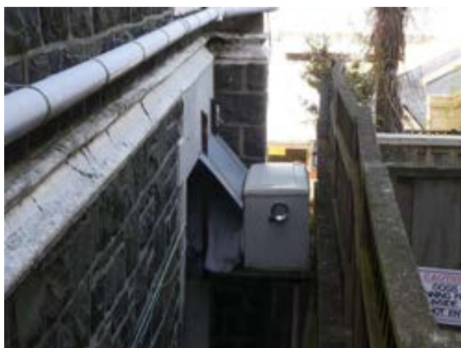
Photograph 253 – Showing the exterior unit of the gas ducted heating system to the western elevation.
