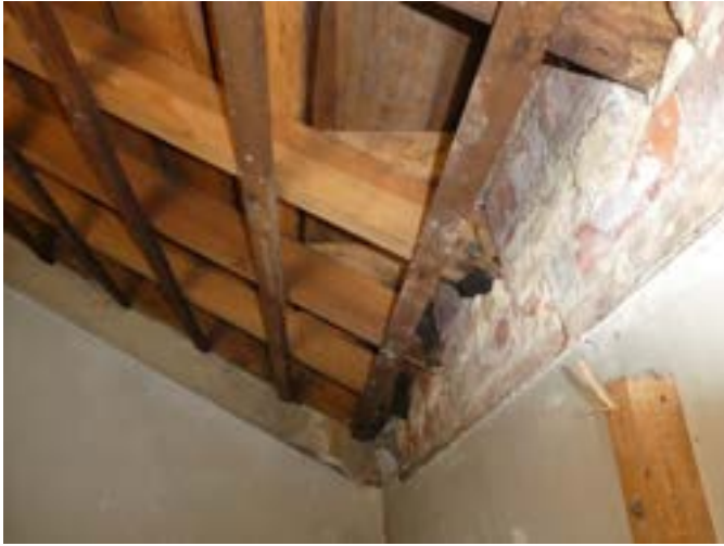
Photograph 118 - Showing the timber rafters built into the solid brick external walls to the western wall of the north western stairwell.
