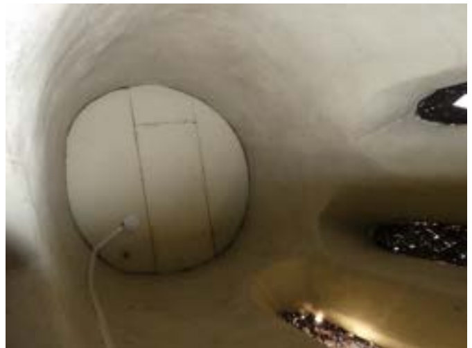
Photograph 157 – Showing the ceiling and sprinkler installed within the bell tower.
