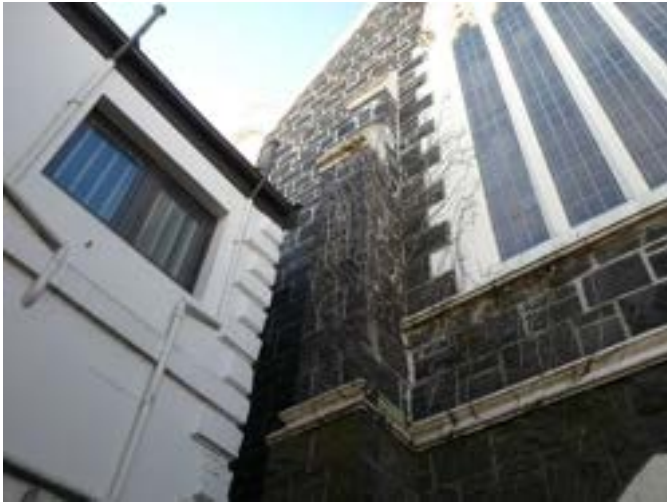
Photograph 33 – Showing the vegetation growth to the western courtyard area.
