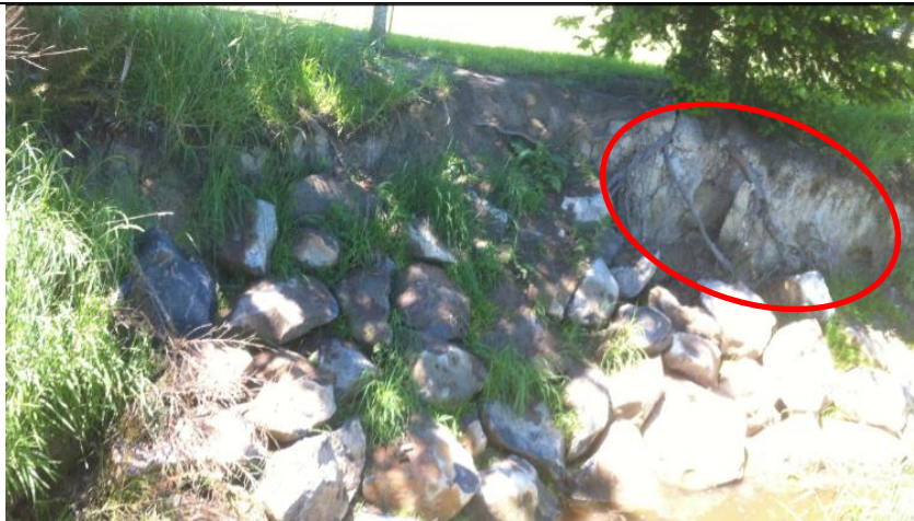
Above: Scouring of the drain, resulting in tree roots left exposed (red circle). Photo taken from submitters property, looking towards the applicants property.
