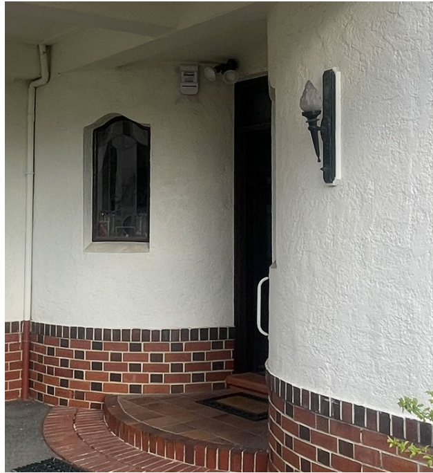
The secondary motor entrance with a typical exterior light fitting.
