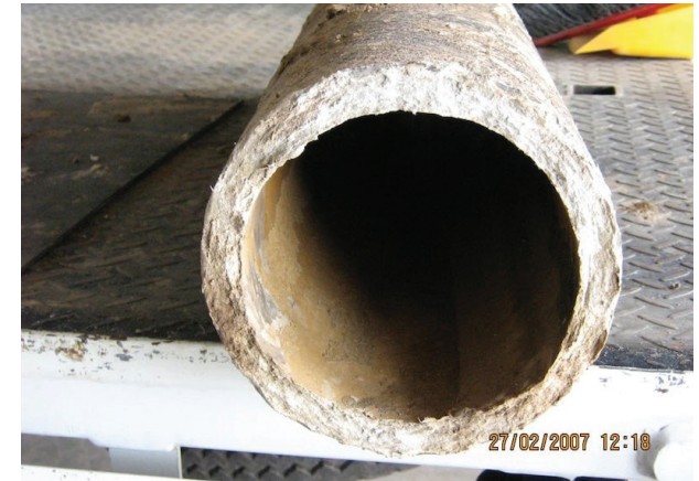
Asbestos containing cement pipe
