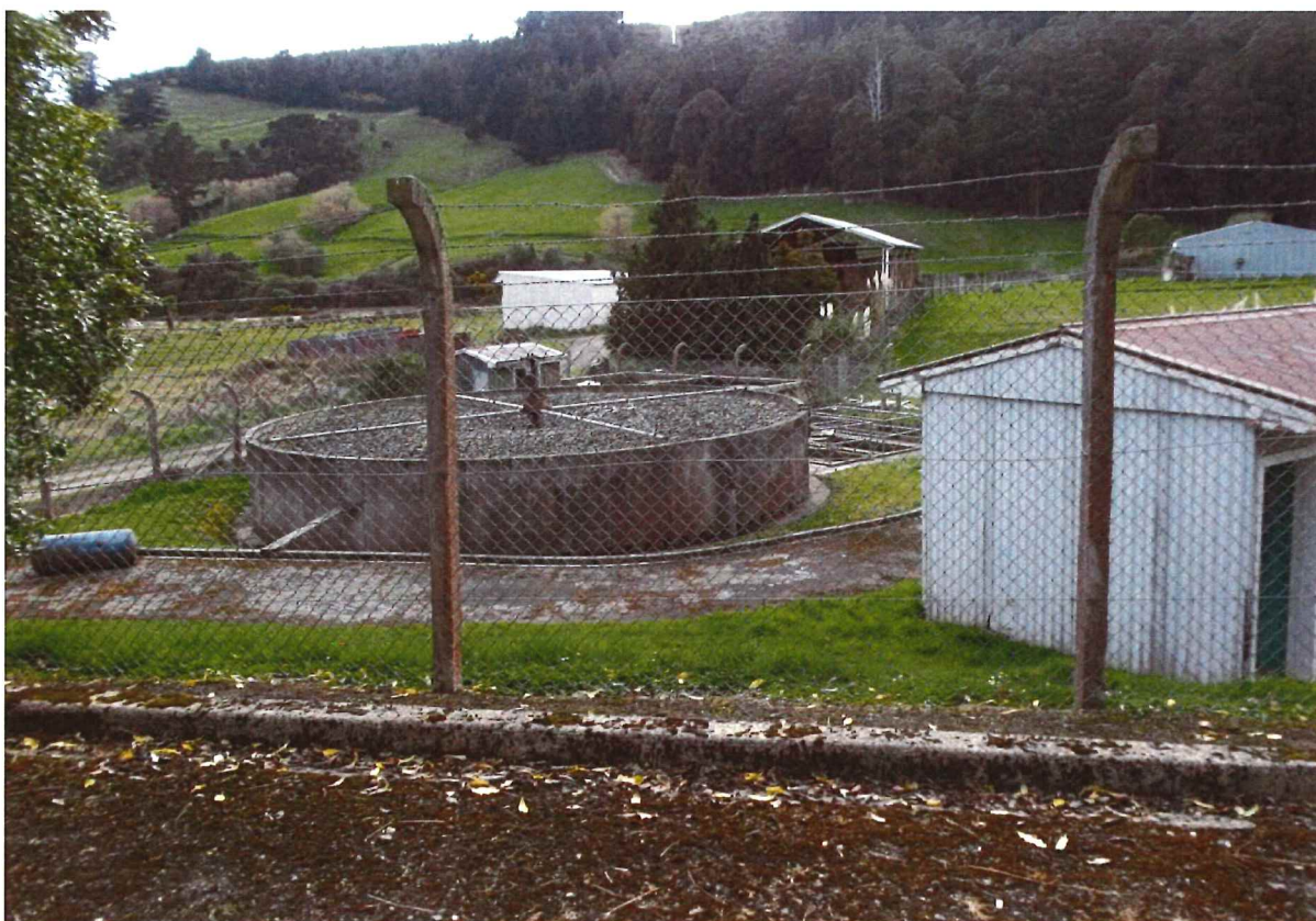
Photo 19: The shared wastewater treatment infrastructure.
