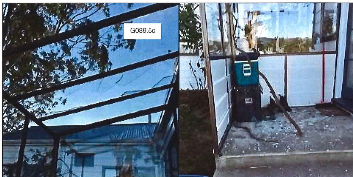
Recent damage to the back porch at 8 Scotia St caused by deadwood falling from the tree shown above left. Evidence of repair costs may be produced if required
