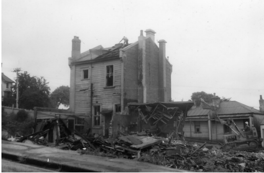
Demolition of dwellings in Perth Avenue during the clearance of substandard housing in 1969 (DCC Archives, https://digitalnz.org/records/37969806/13-perth-avenue-from-palmyra-street-during-demolition-17-december-1969 )
