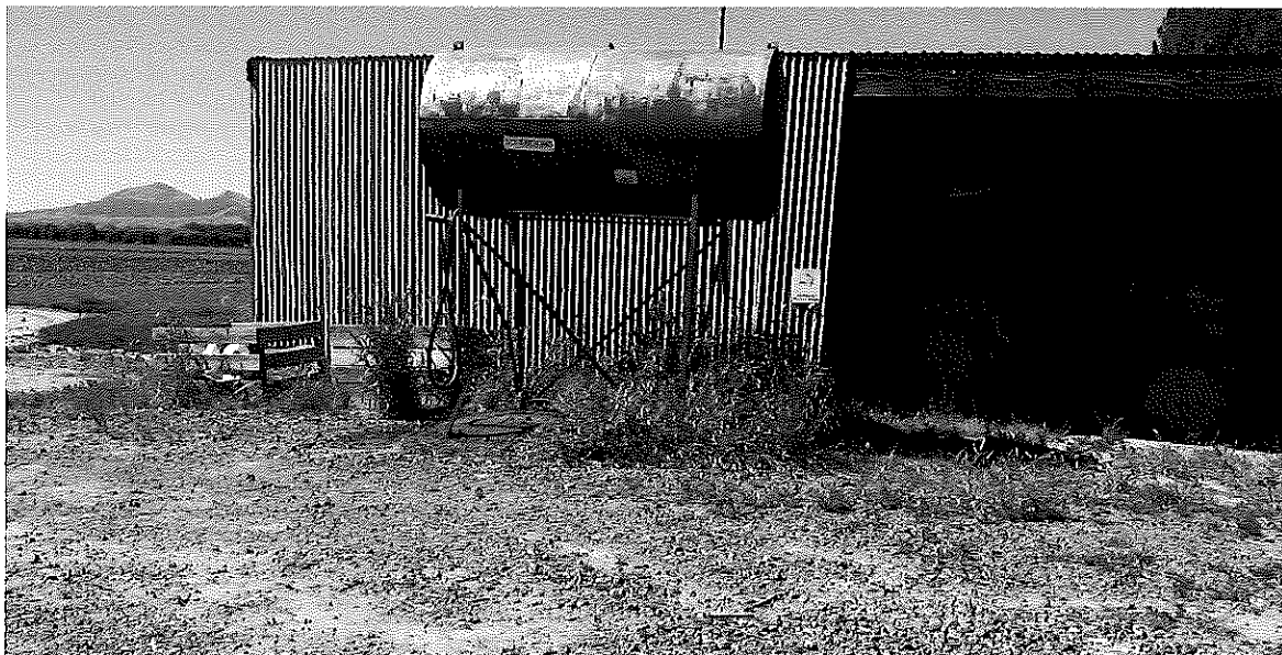
Figure 14: Diesel tank beside tractor shed at 498 Allanton Road. The tank is not bunded and localised diesel staining is evident in the ground at the base of the tank stand. Two bins for storing plastic rubbish prior to disposal are located beside the tank stand.
