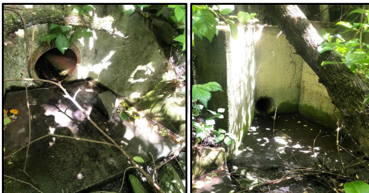
Figure 7: Stormwater discharge pipes at boundary of 177 Tomahawk Road, with untreated stormwater flowing to a soak hole.
