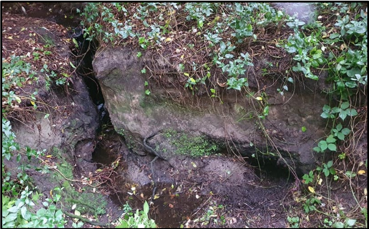
Figure 8: Stormwater erodes the hillside and enters a deteriorated soak hole where it flows into a 30 cm wide hole within 177 Tomahawk Road.
