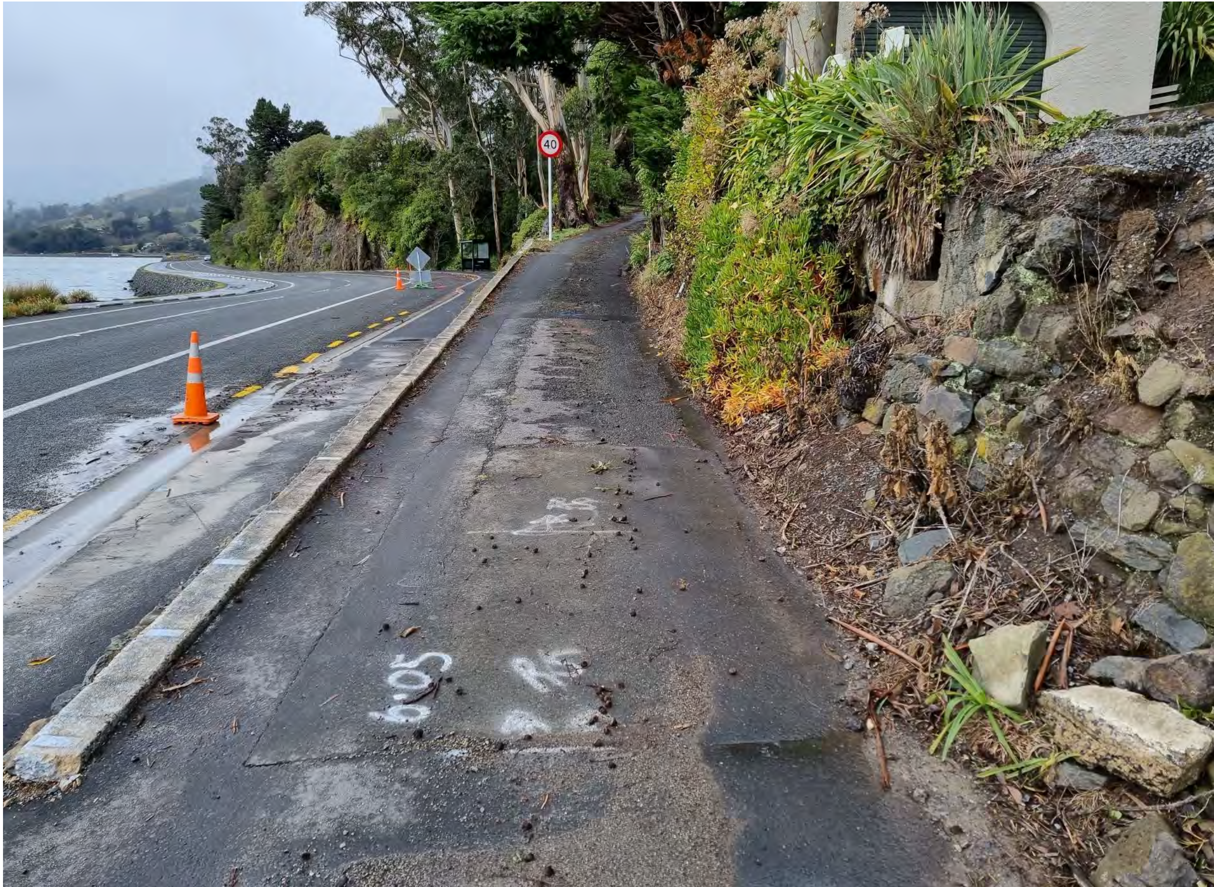
ATTACHMENT C.5 PHOTO 1 OF Weller Street uneven surfacing, and rutting and ravelling of the surfacing observed
