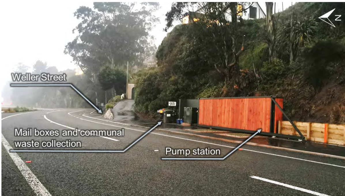
Figure 11 New pump station on Portobello Road beside Weller Street
