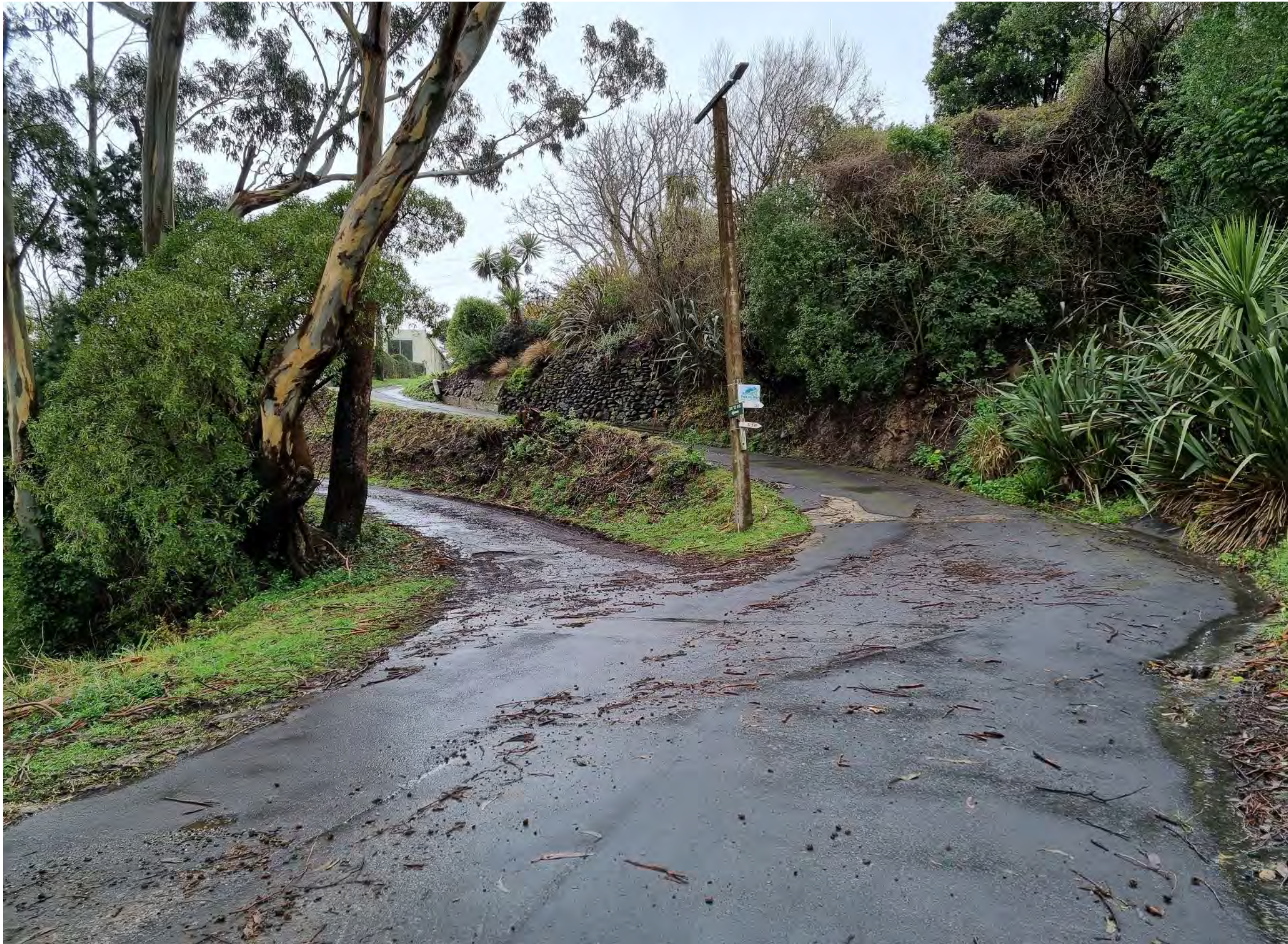
ATTACHMENT C.6 PHOTO 2 OF Weller Street uneven surfacing, and rutting and ravelling of the surfacing observed
