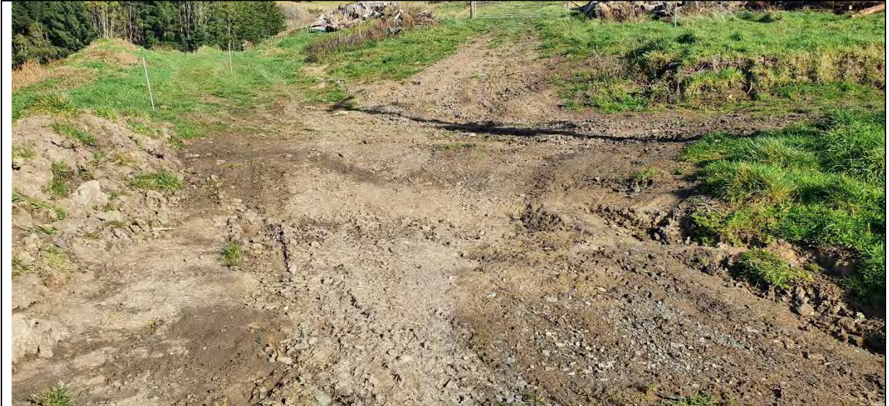
Plate 5: View at intended upper roundabout location where three farms track intersect, with little erosion noted.
