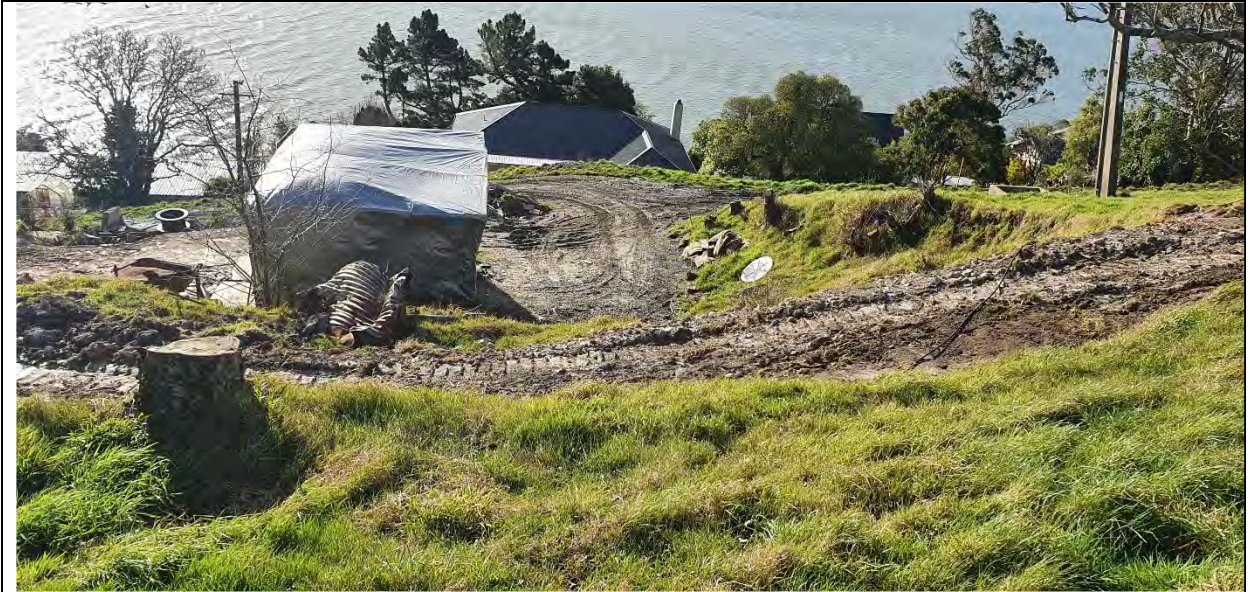
Plate 4: Looking down on demolished house site with over steep formed slopes and non-engineered fills at front.
