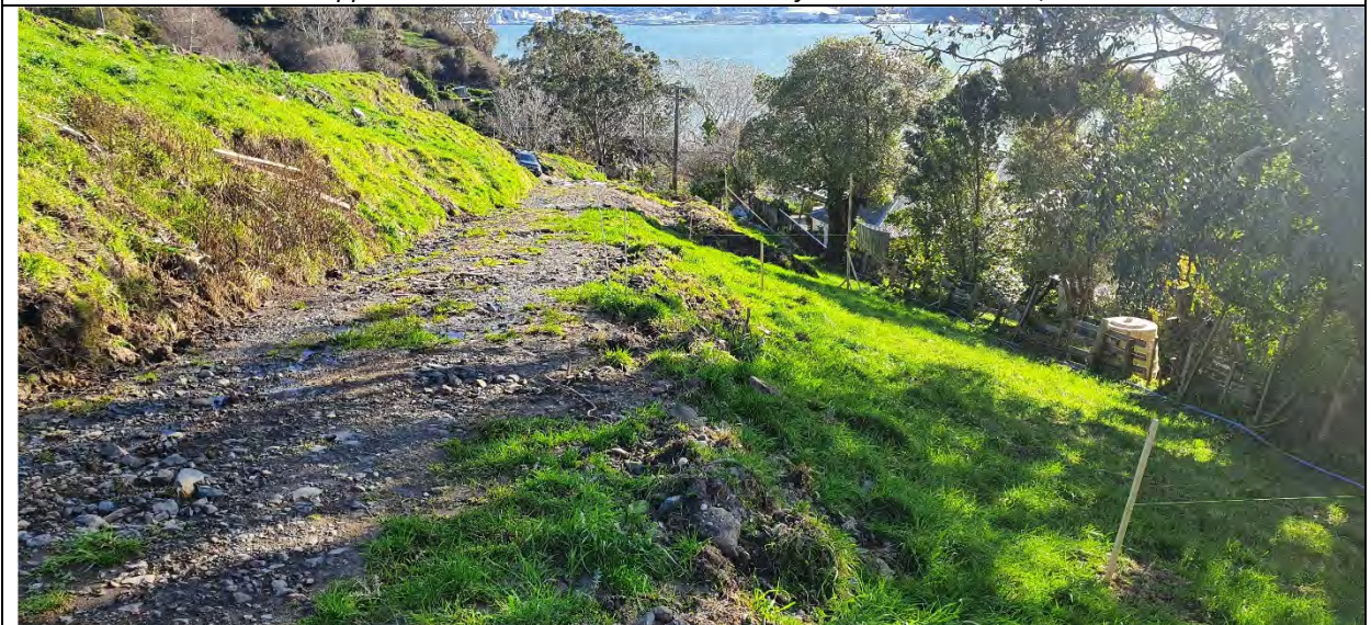
Plate 5: Looking down the lower farm track (GHD ch250) with existing steep non-engineered fills on side slopes
