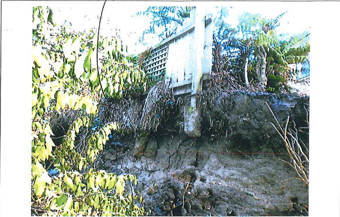
Photograph 3: View of scour from flood flow in the creek
