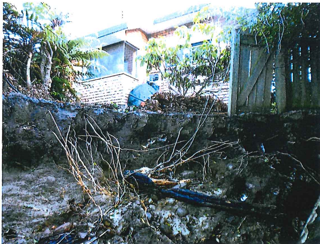
Photograph 4: View of scoured area from the creek
