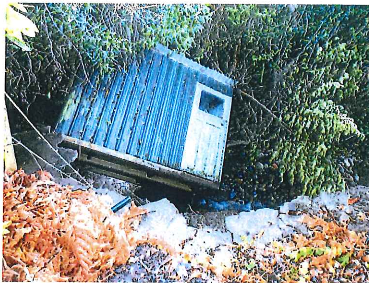
Photograph 1: View of the scour damage from the top of the slope showing shed in creek
