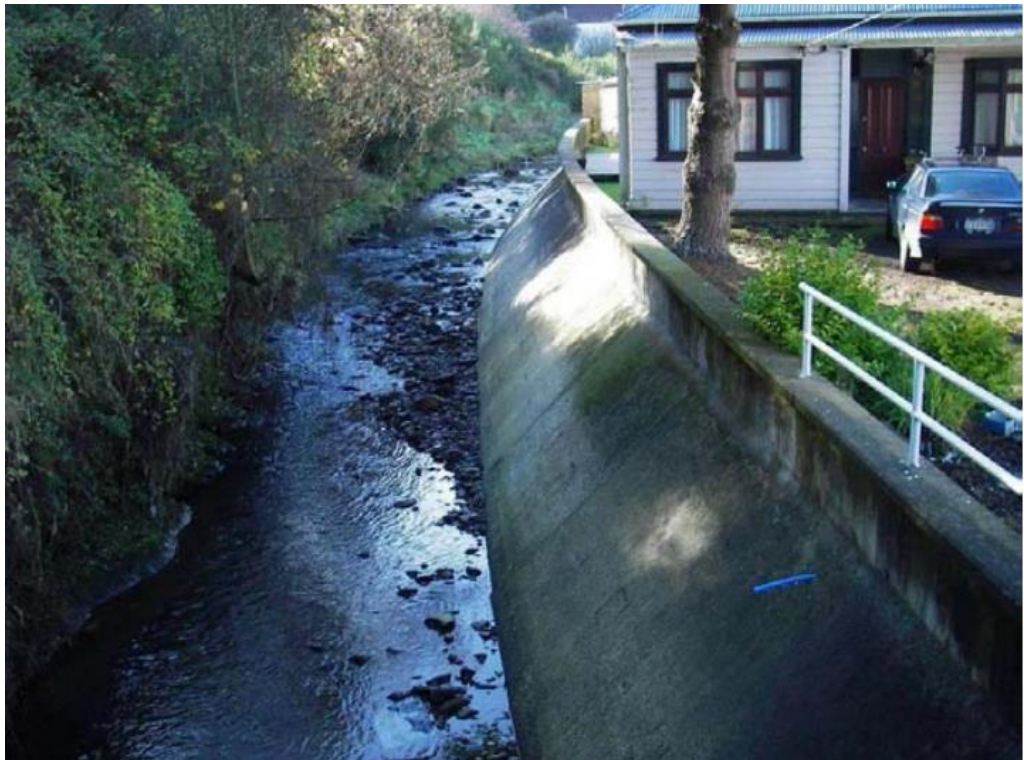
Figure 7. Example of a narrow section of Lindsay Creek and house located immediately next to the main channel of Lindsay Creek
