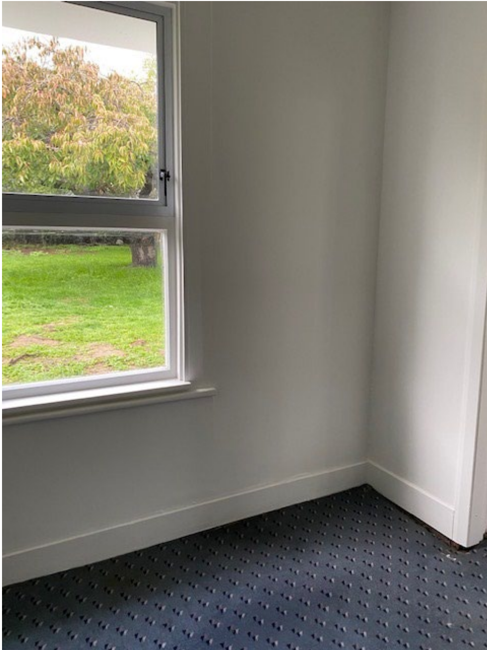
Image 5: Internal front room, floor deteriorating
