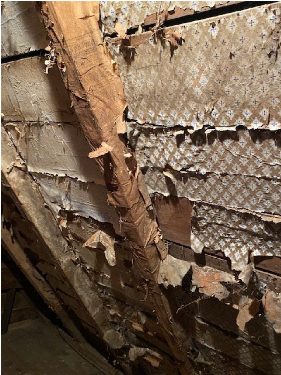
Image 7: Attic: demonstrating old wallpaper and newspaper lining, proof of habitation of attic
