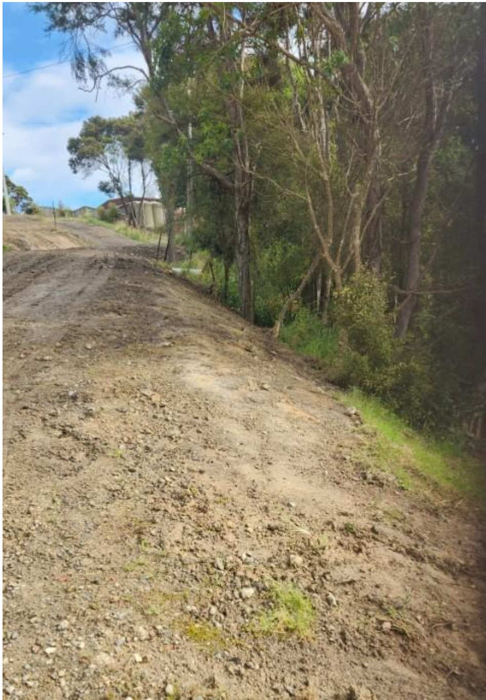
Photograph 6: Road shoulder following removal of all (recent) fill (photo supplied by P Napier)
