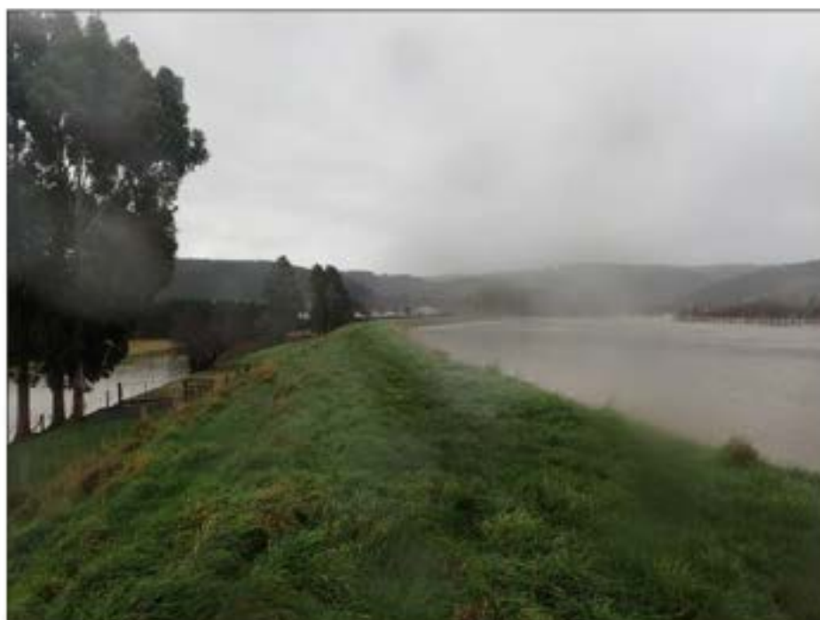
Photograph 1: View North Along Flood Bank (2017 Flood Event)
