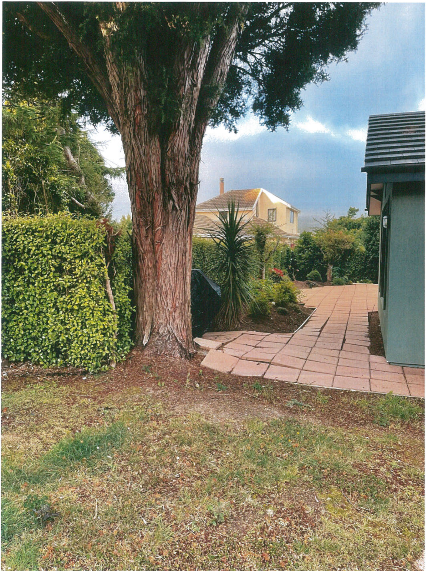
Image 2- Damage to ground profile and pavers
