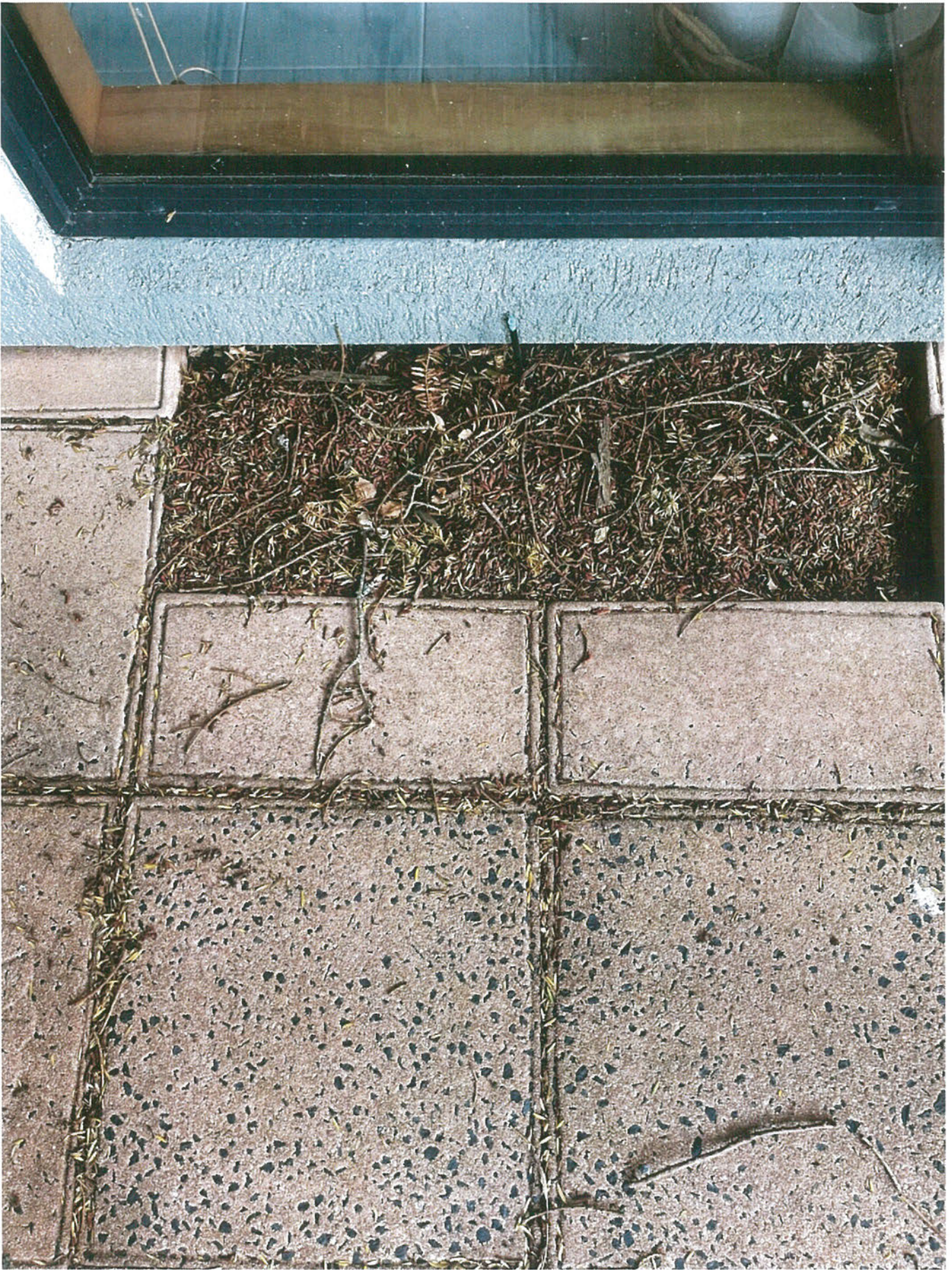
Image 4- Drainage sump blocked by needles
