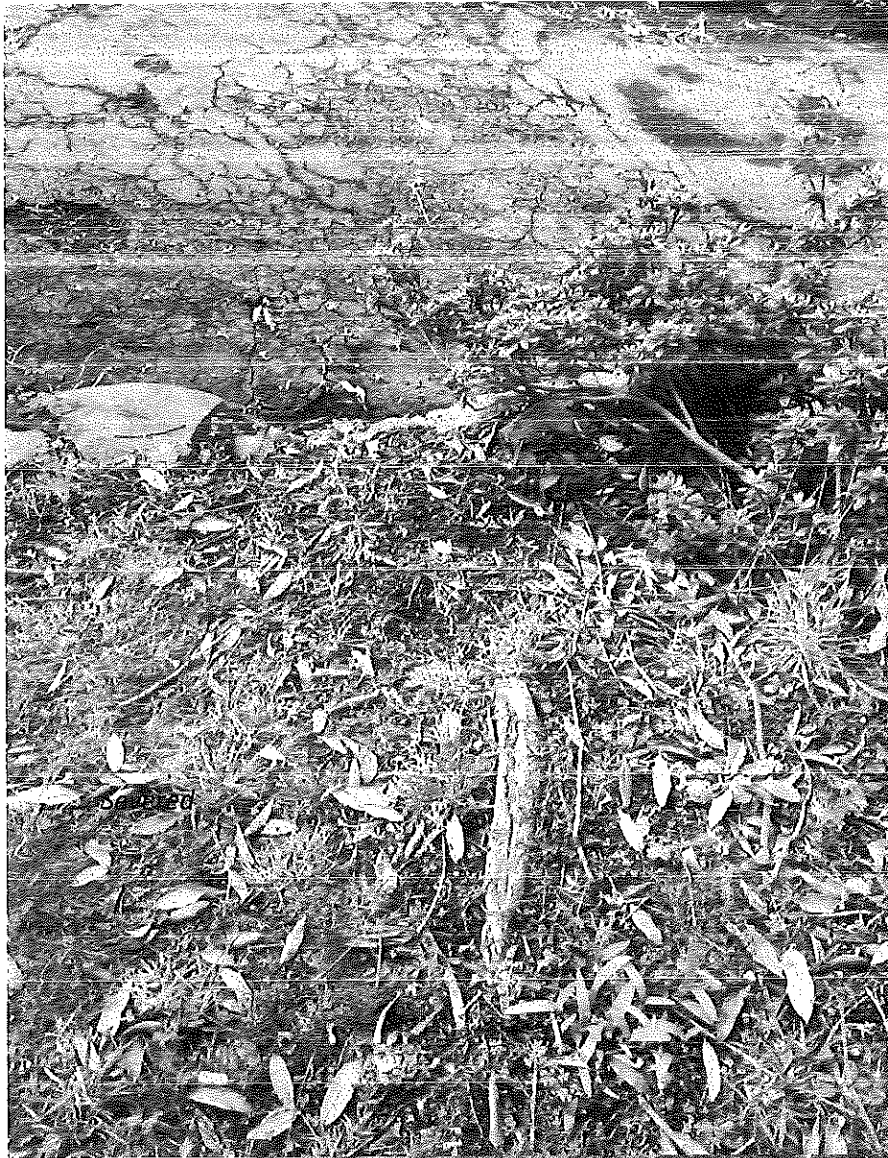
Exposed roots northern side of tree
