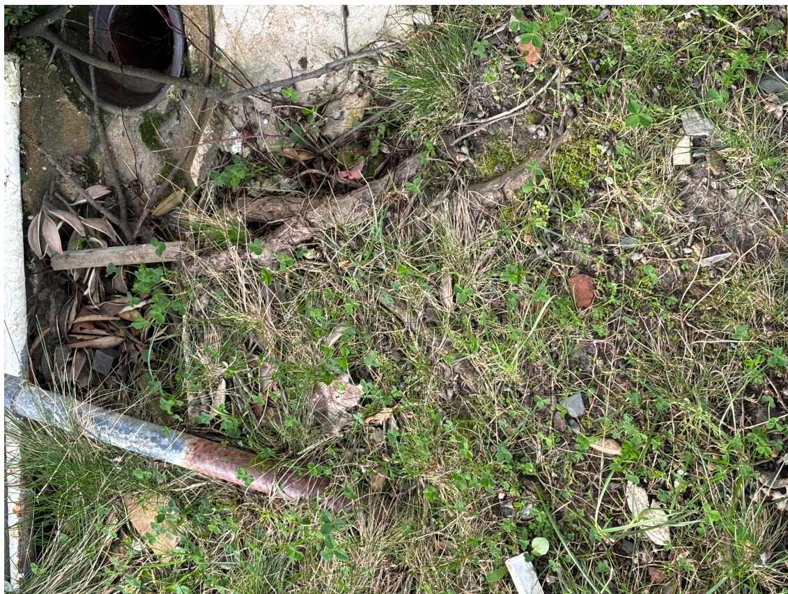
Image two: Image showing the top of the stormwater pipe where the down-pipe (not visible) connects with the stormwater drainage system. Surface roots can be seen running towards this junction.
