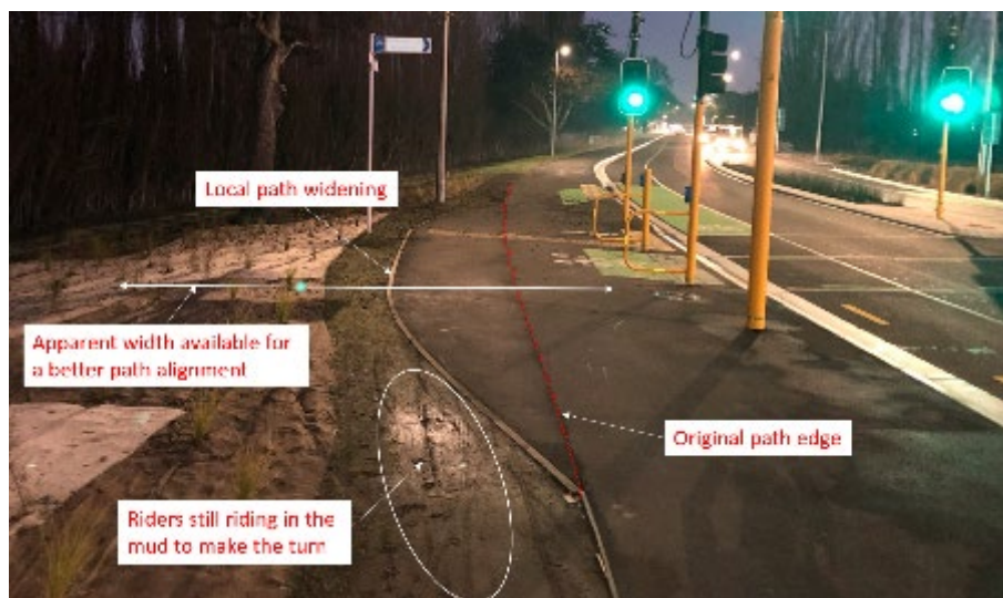
Figure 2-4: poor post construction fix for right angle turns in parallel paths
