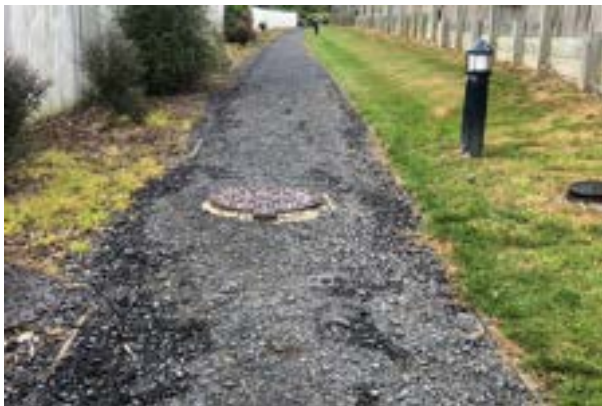
Figure 2-2: protruding path hazard
