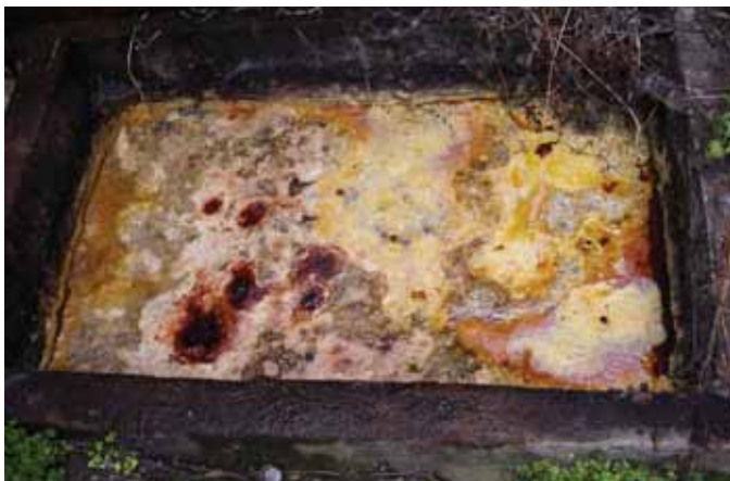
Poorly maintained grease trap
