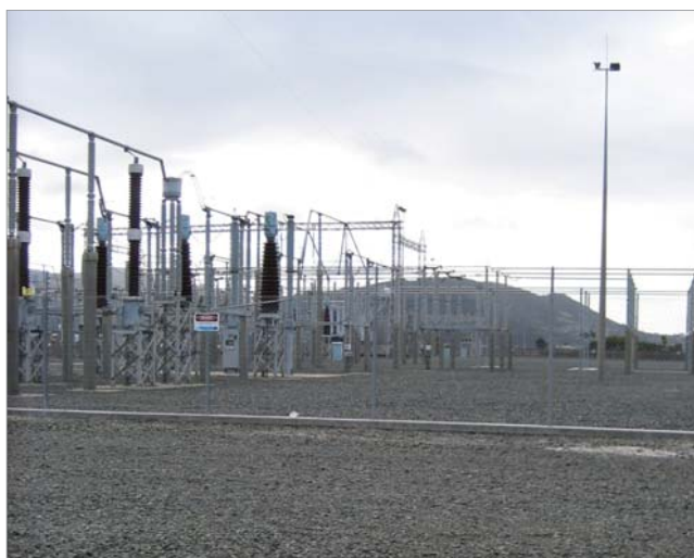
Power Substation on Otaki Street
