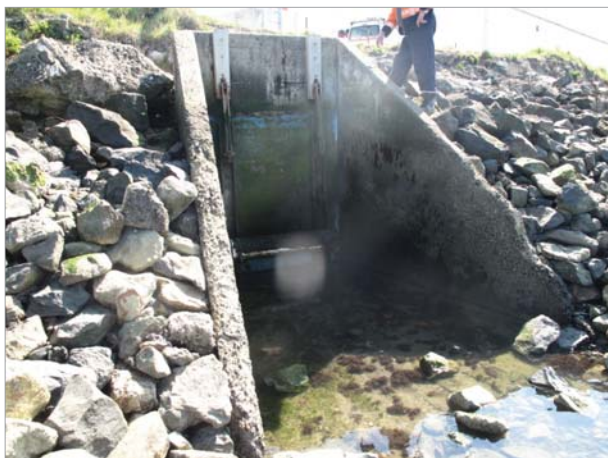
Catchment Harbour Outfall at Kitchener Street
