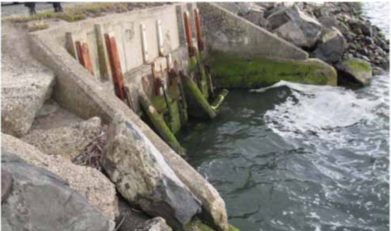
Figure 5-1: Orari Street Stormwater Catchment Outfall
