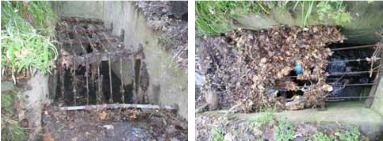
Figure 8-2: Intake at 91 Glen Road
