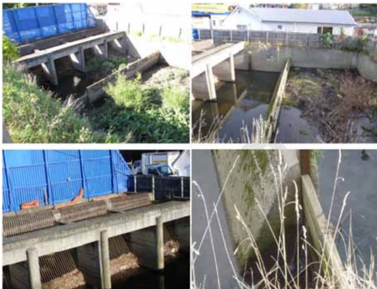
Figure 4-9: Glen Intake Structure, Including Weir and Screens
