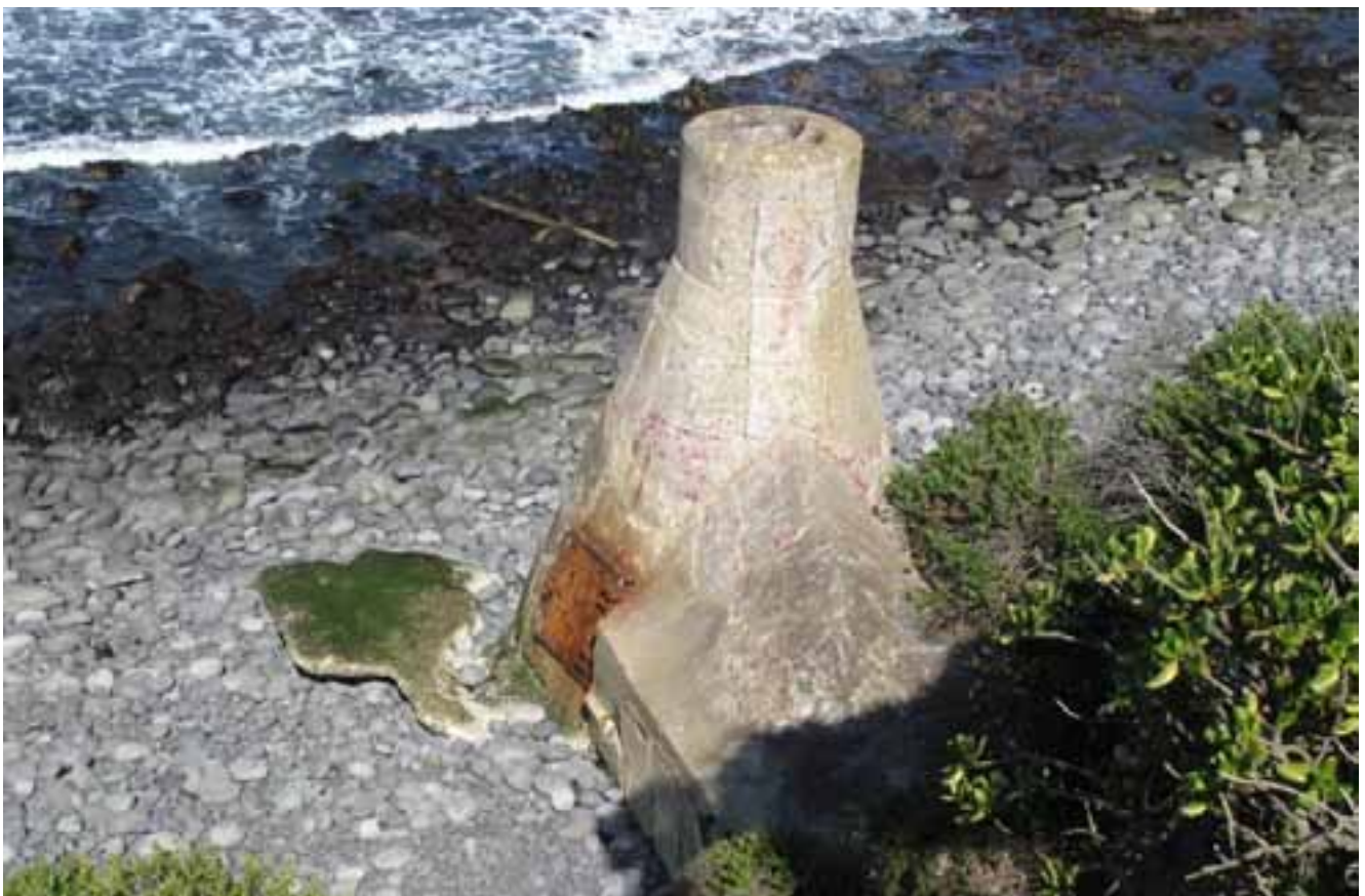
Figure 5-1: St Clair Catchment Bell Chamber Outfall at Second Beach
