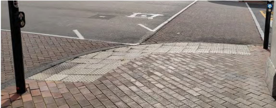
Figure 26: Barnes Dance Crossing St Andrews Street – Incorrect TGSI configuration and uneven surface 20
